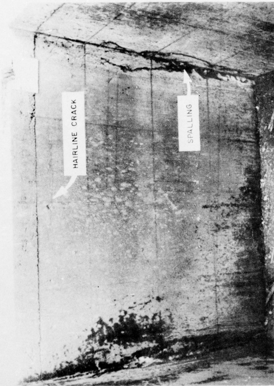
Fig 13 Post-test damage to Cell No. 1 east wall (Test No. 4)
