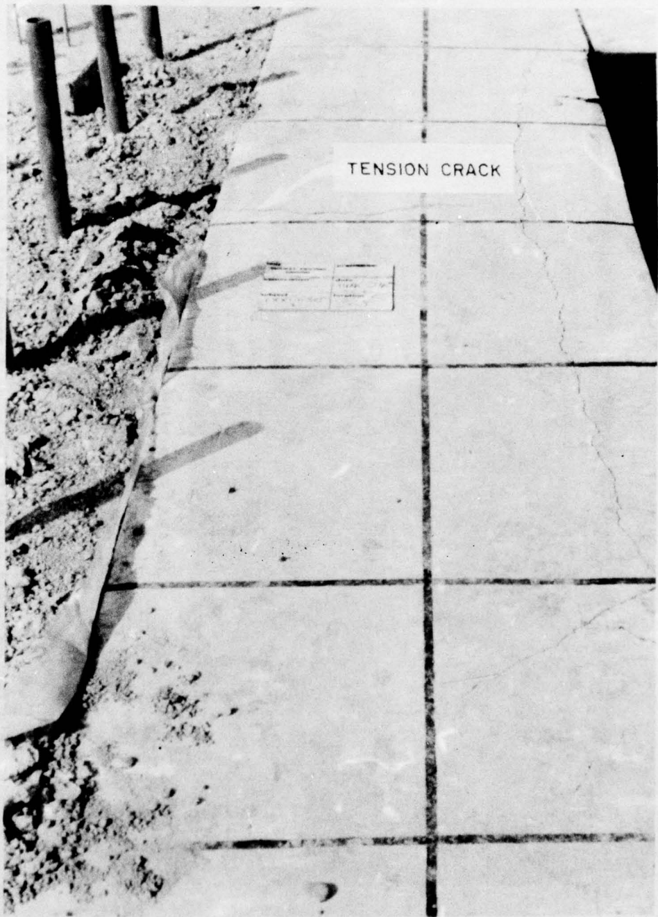
Fig 17 Post-test damage to Cell No. 1 apron (Test No. 5)
