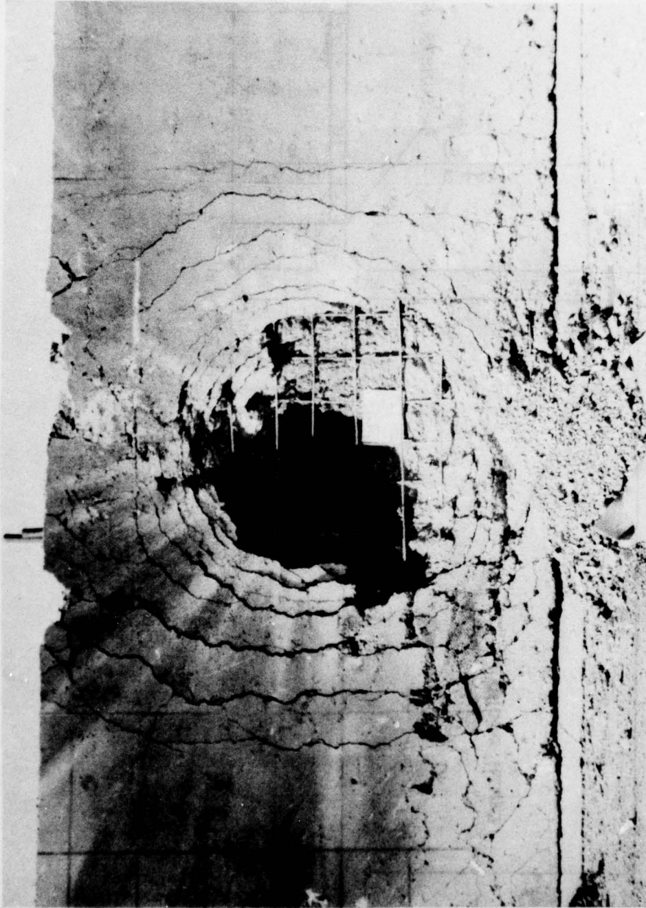
Fig 64 Post-explosion view of Wall No. 1 - Barricade Tests
