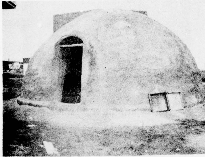
Figure 10(b). Completed 28-ft (8.5-m)-diameter by 14-ft (4.3-m)-high steel fiber shotcrete dome. The dome consists of 6-in (.15-m)-thick polyurethane foam and 2 to 3 in. (.051 to .076 m) of 1.5 volume percent steel fiber shotcrete.
