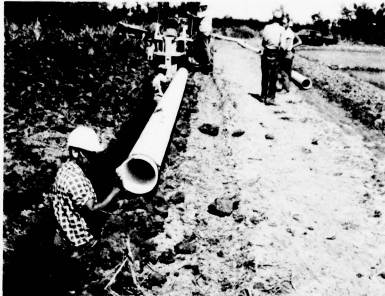
Underground pipe is used in some cases as part of the on-farm distribution system.
