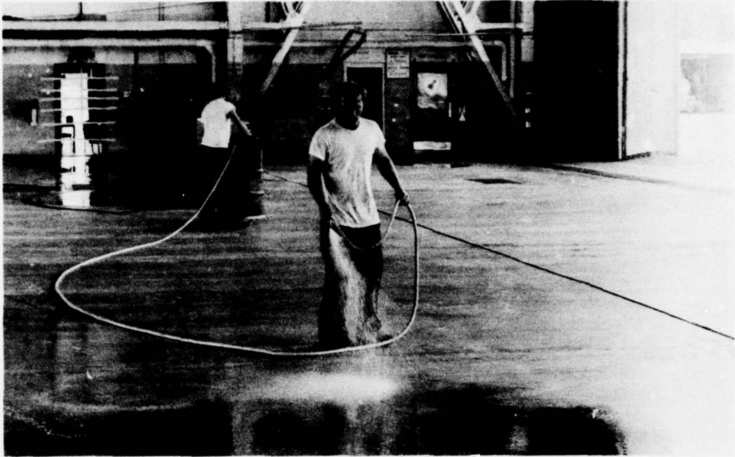
Figure 2. Application of cleaner-remover high flash naptha solvent to deck to remove grease and oil.
