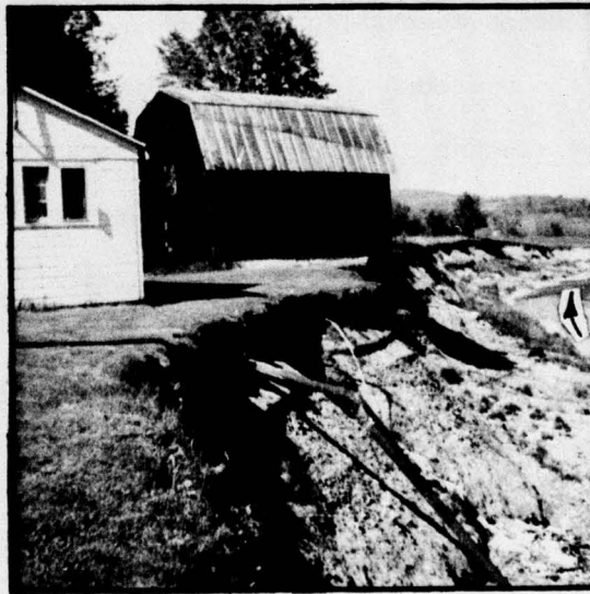
Photo No. 14 - Bank erosion on an outside river bend along New York route #19, just south of the village of Belfast which is seriously endangering a house and barn. The state of New York is planning bank stabilization work in this area to protect route #19. Photo was taken in May 1966.
