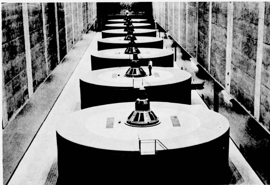
Figure 4.7 Generator Room, Clark Hill Powerplant, Where 700 Million Kilowatt-Hours Are Generated Annually.
