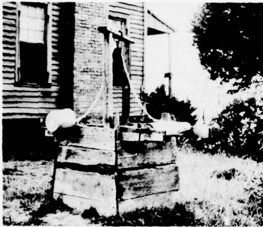
Figure 2.3 Substandard Wells Require Improved Construction with Proper Sealing to Protect Domestic Water Supplies.
