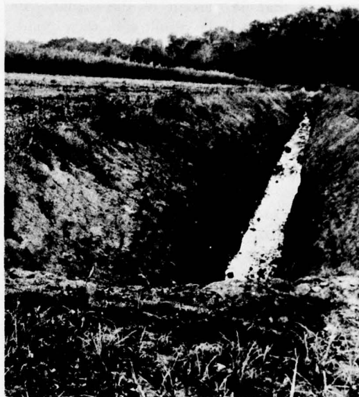
Figure 2.9 Drainage Project, Thomas County, Georgia—Drainage Offers Extensive Opportunities.
