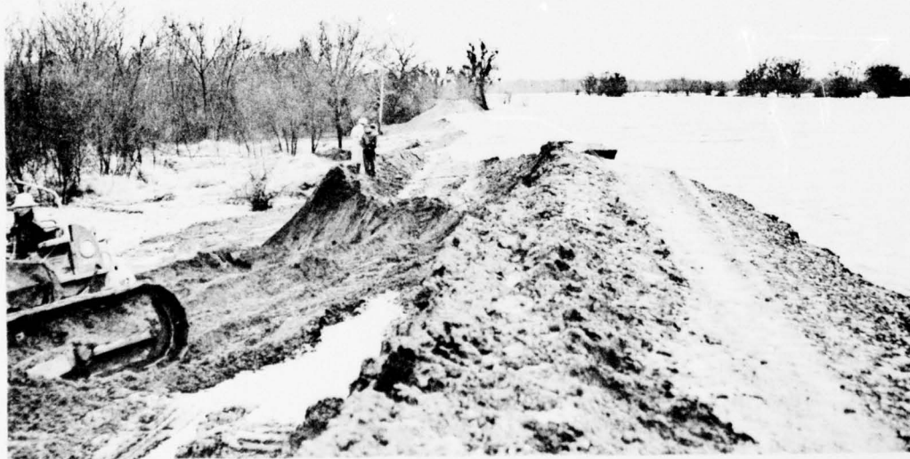
Ten minutes later, however, the levee was breached and floodwaters began to flow.
