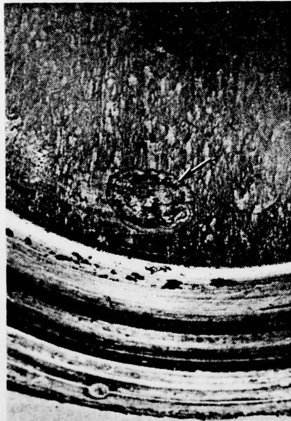
Figure 18. Corrosion in Housing, Main Junction Box (Enlarged)
