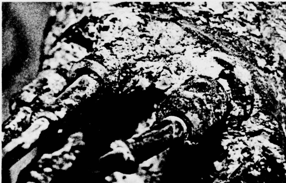
Figure 3. Exterior Corrosion, Junction Box, Array 7 (Approx. life size)
