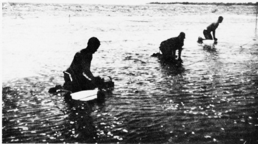
Seagrass transplanting operation on dredged material near Port St. Joe, Florida. In the absence of mechanized techniques, seagrass transplantation is now a labor-intensive effort.
