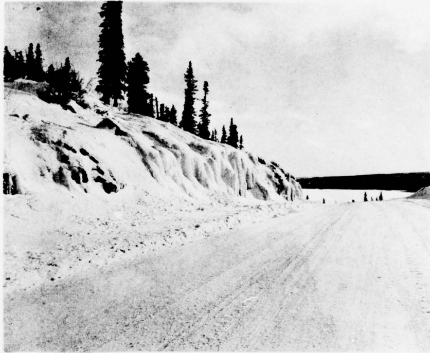
Figure 5. Water seepage down the face of this cut slope in rock has frozen and completely filled the ditch between the cut face and the road.
