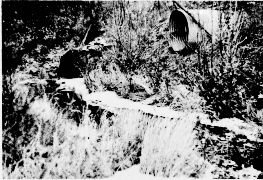
Figure 9. A staggered culvert installation. The upper culvert at right can carry flow when the lower culvert is blocked by ice.
