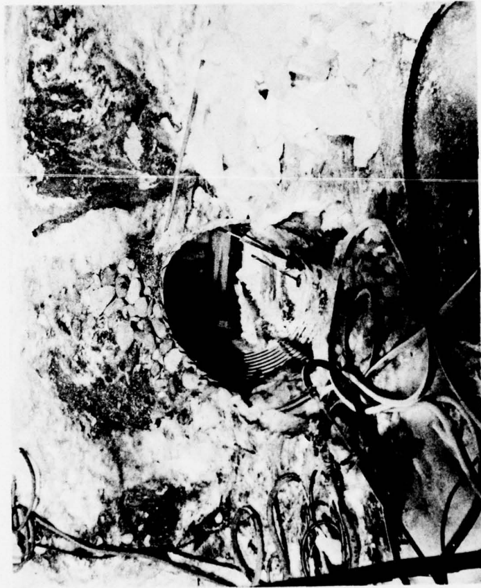
Figure 1. An ice-filled culvert being cleared by steam and hand tools to prepare for spring runoff.
