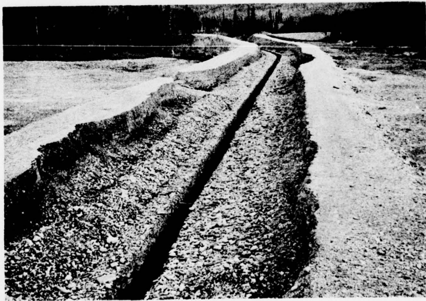
Figure 10. A specially-constructed narrow deep channel to carry low winter flows. The narrow channel is formed by rock-filled wire gabions.
