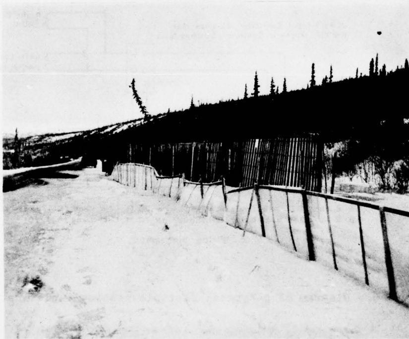
Figure 8. An ice fence installation, which is holding back ice formed by seepage from the slope at right.
