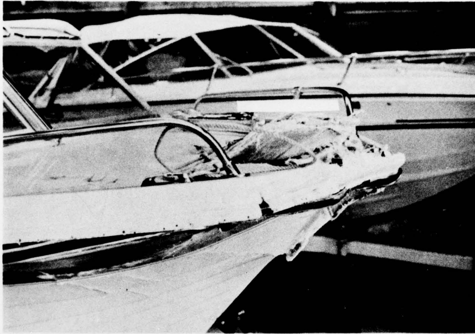
FIGURE 5. STRUCTURAL DAMAGE TO BOW (STARBOARD SIDE VIEW)
