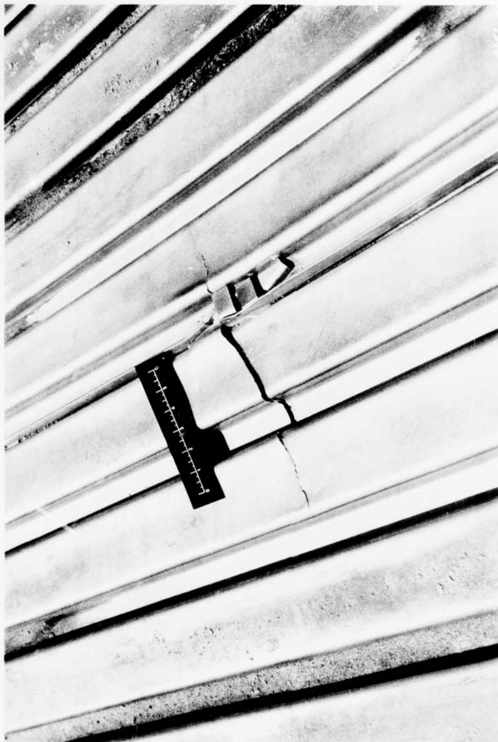
Photo 19. Split in Fletcher panel 43 after 3000 passes
