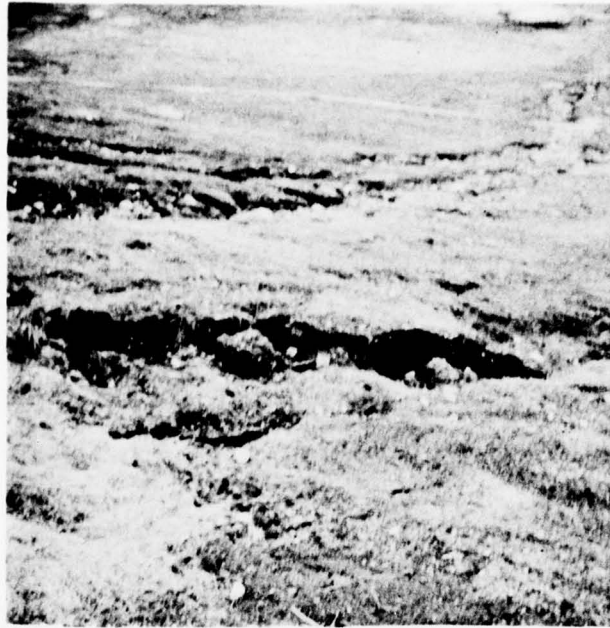
Figure 16. Erosion ditches caused by running water from the adjacent parking lot.
