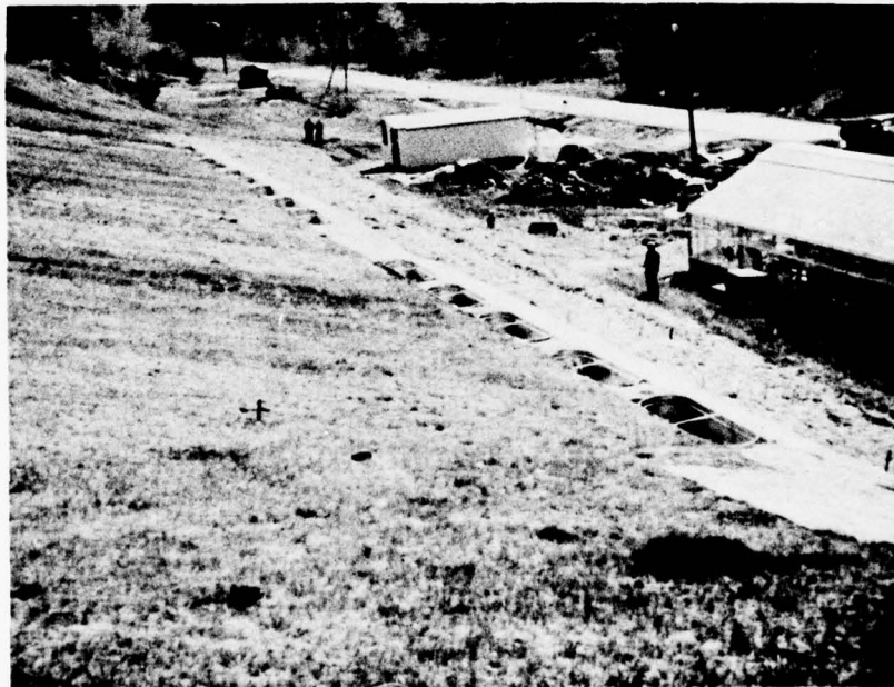
Figure 9. Final tank installation. Note jute net around tanks for erosion control during construction.
