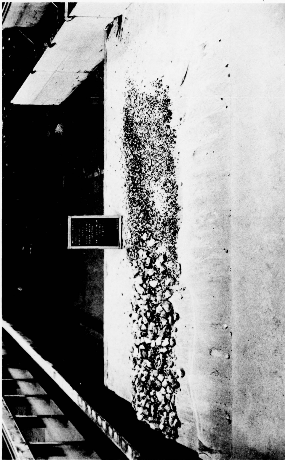
Photo 6. Sea-side view of Plan 2 in the deeper water location after 1.0 hr of 14.0-sec, 12.1-ft waves at an swl of +5.4 ft mllw
