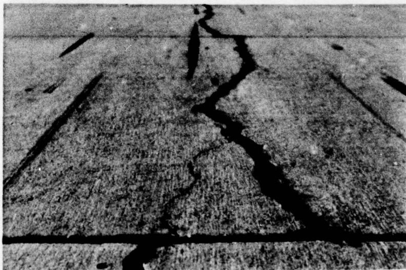
Figure 86. High Severity Longitudinal Cracks.
