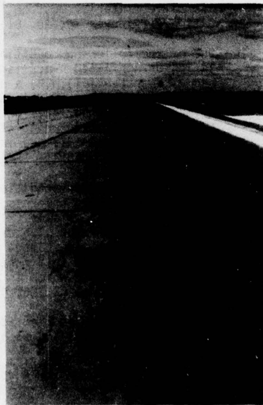
Figure 80. Low Severity Filled Longitudinal Cracks.
