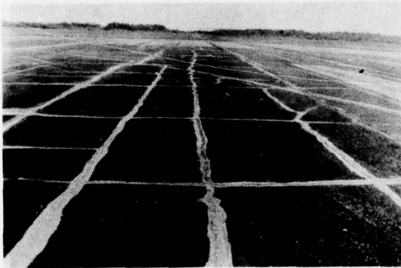
Figure 14. Low Severity Block Cracking, Filled Cracks.
