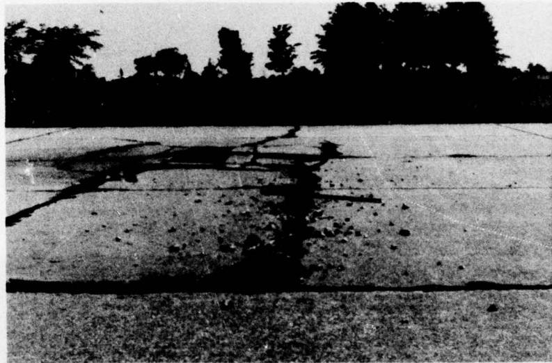
Figure 71. Low Severity Blow-Up. (Note That This Would Only Be Considered Low Severity If the Shattering in the Foreground Was the Only Part Existing and the Foreign Material Removed.)
