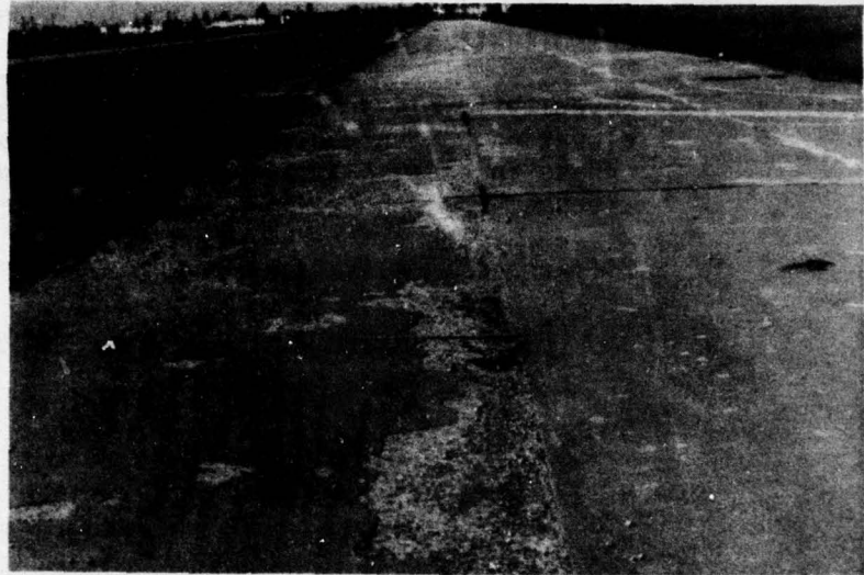
Figure 113. High Severity Scaling.
