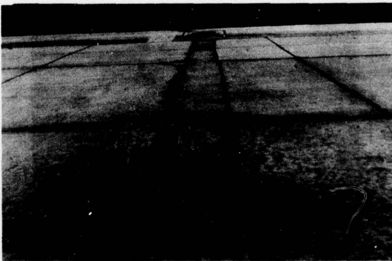
Figure 103. Low Severity Utility Cut.
