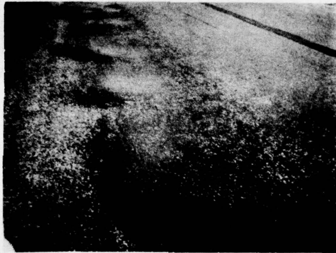
Figure 24. High Severity Corrugation.
