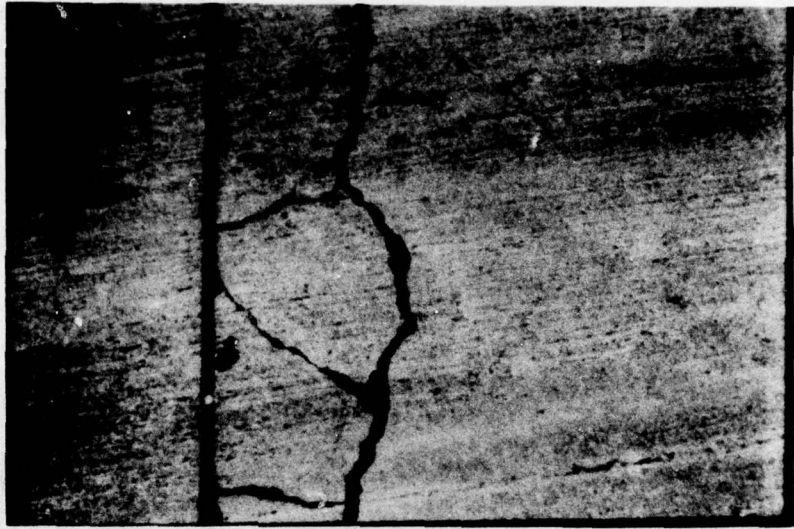
Figure 132. Medium Severity Joint Spall.
