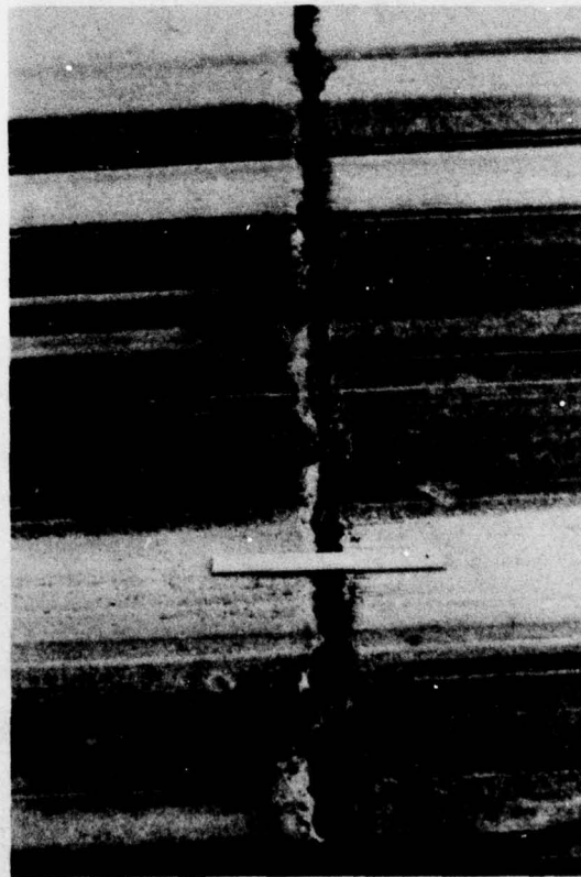
Figure 129. Low Severity Joint Spalling. (If the Frayed Area Was Less Than 2 Feet Long It Would Not Be Counted.)
