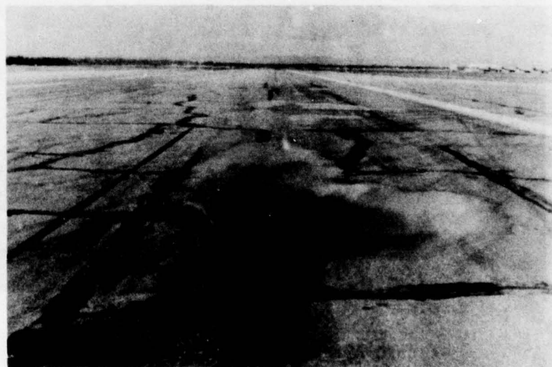
Figure 28. High Severity Depression (2 Inches).
