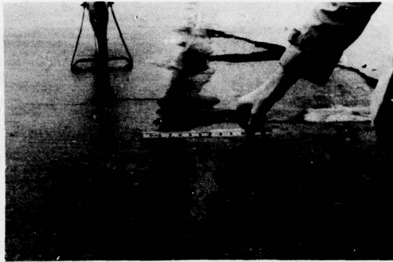
Figure 117. Medium Severity Settlement on Apron (>1/2 Inch).
