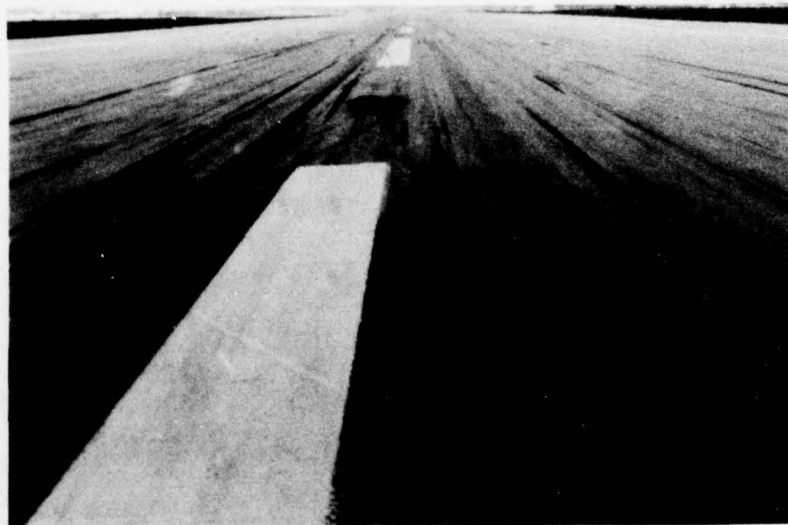
Figure 29. Jet Blast Erosion.
