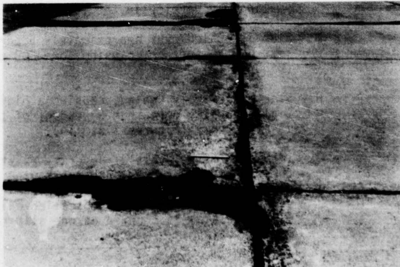
Figure 112. Medium Severity Scaling.
