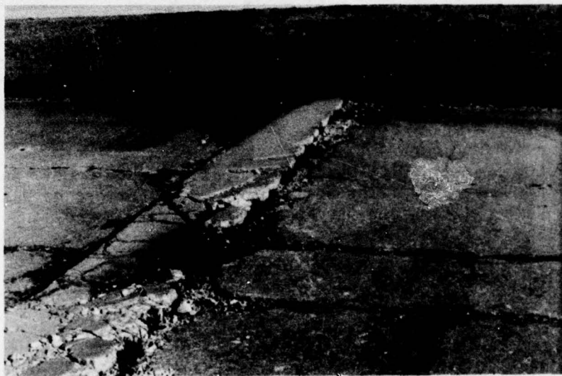
Figure 73. High Severity Blow-Up.
