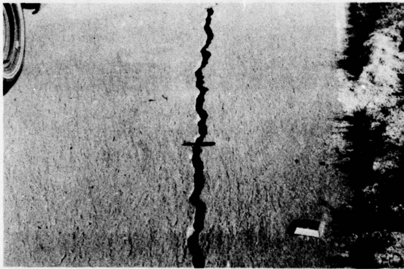
Figure 87. High Severity Crack.
