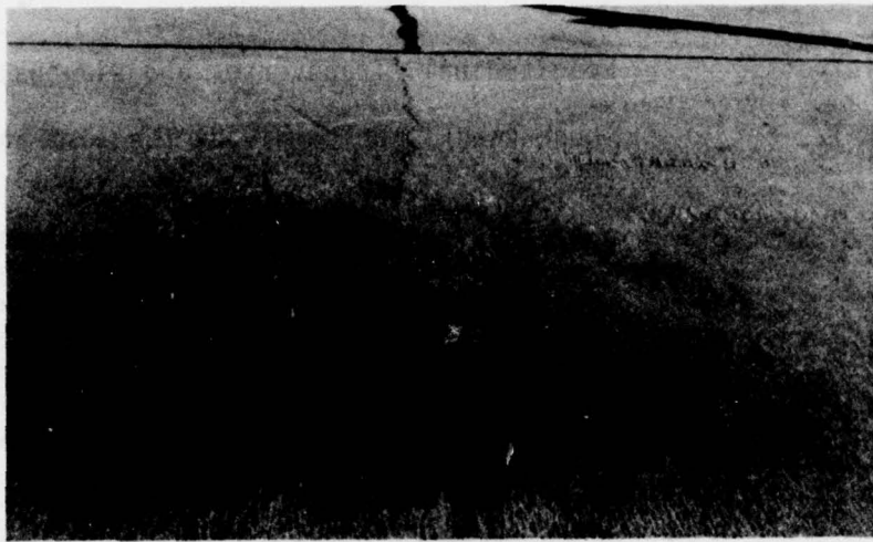
Figure 79. Low Severity Longitudinal Crack.
