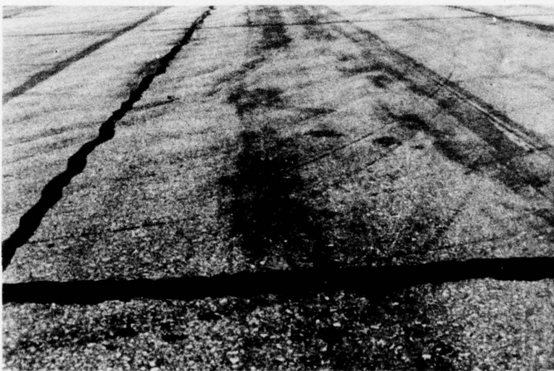
Figure 32. Low Severity Joint Reflection Cracking, Filled Crack.
