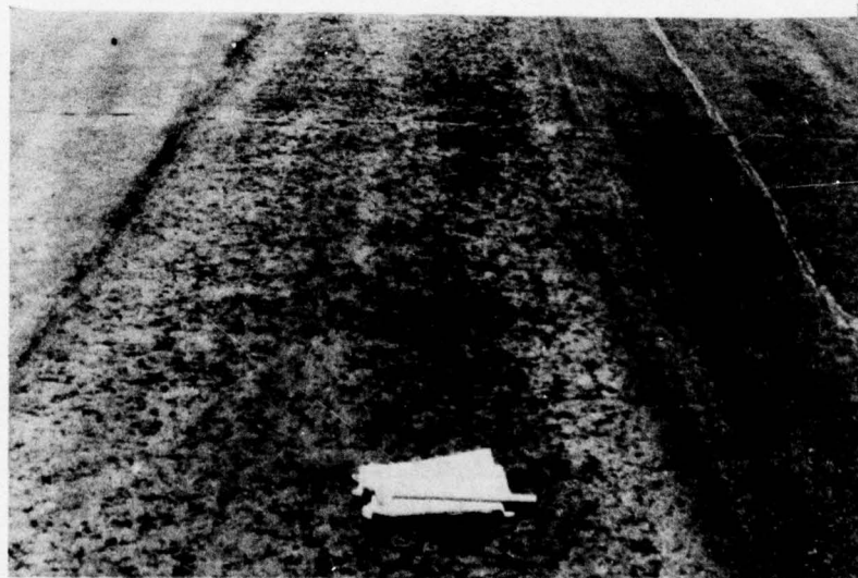
Figure 54. Light Severity Raveling/Weathering, Approaching Medium Severity.
