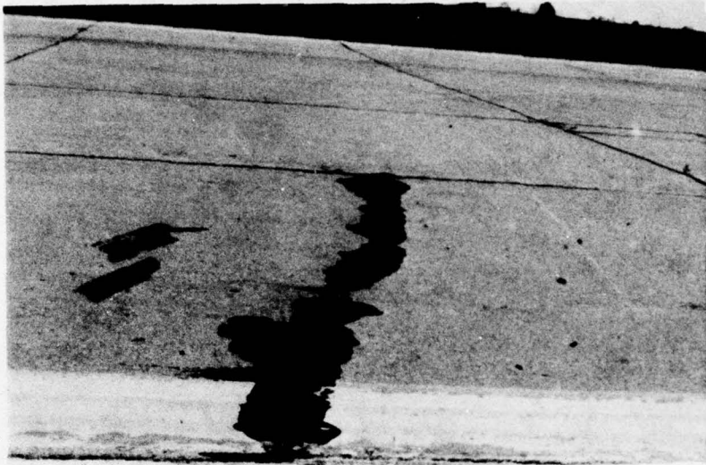
Figure 83. Medium Severity Transverse Crack.
