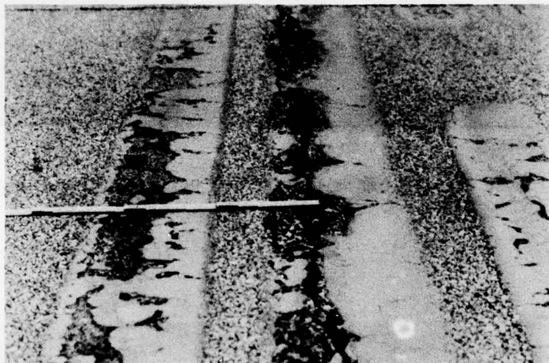
Figure 37. High Severity Joint Reflection Cracking.
