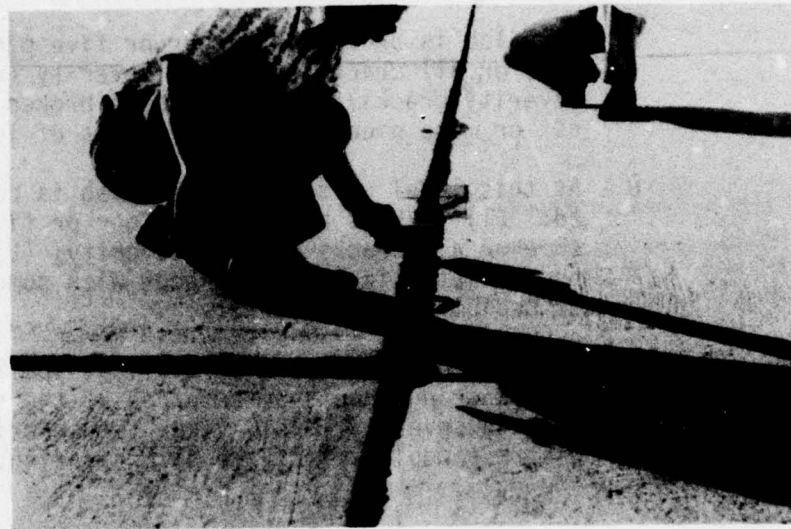
Figure 119. High Severity Settlement.
