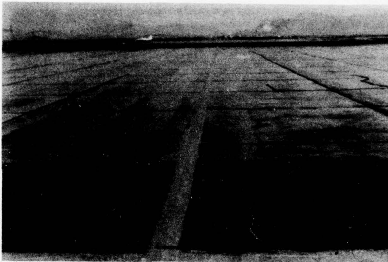
Figure 31. Low Severity Joint Reflection Cracking.
