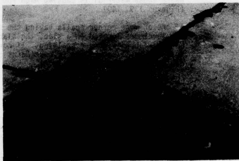
Figure 136. Low Severity Corner Spall.
