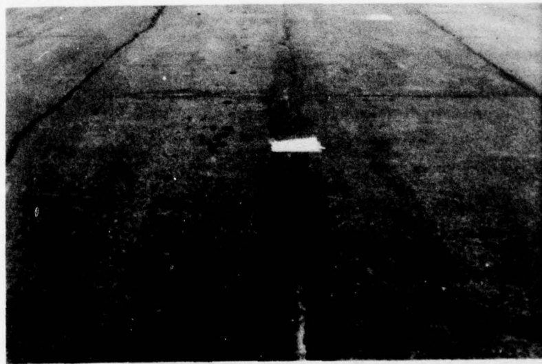
Figure 41. Medium Severity Longitudinal Crack. (Note the Crack Is Reflective But Not at the Joint of Slab.)
