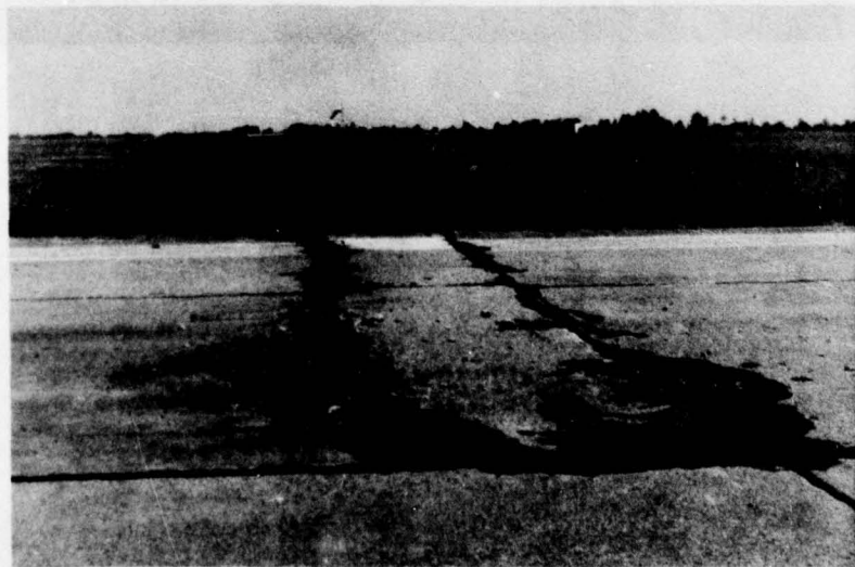
Figure 72. Medium Severity Blow-Up.
