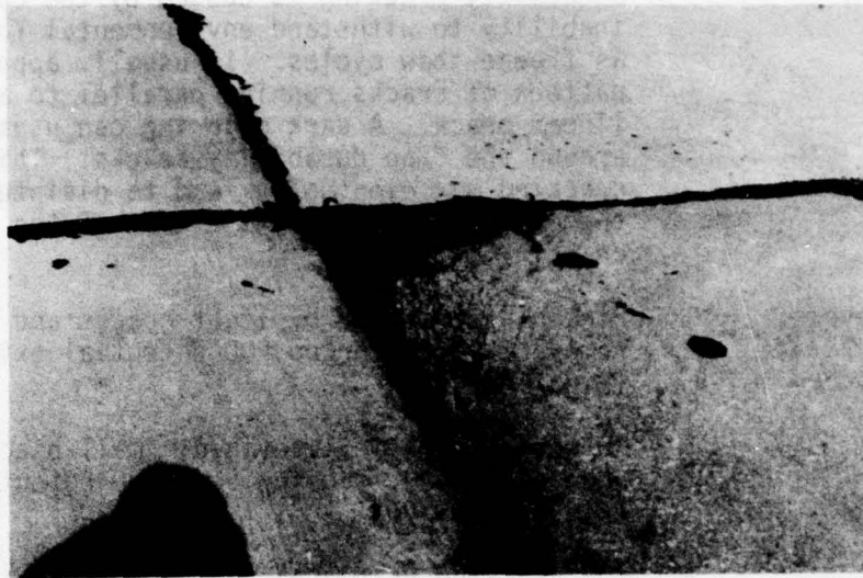
Figure 88. Low Severity "D" Cracking.
