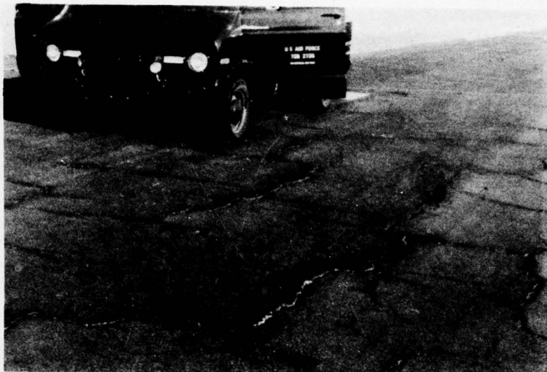
Figure 19. High Severity Block Cracking.
