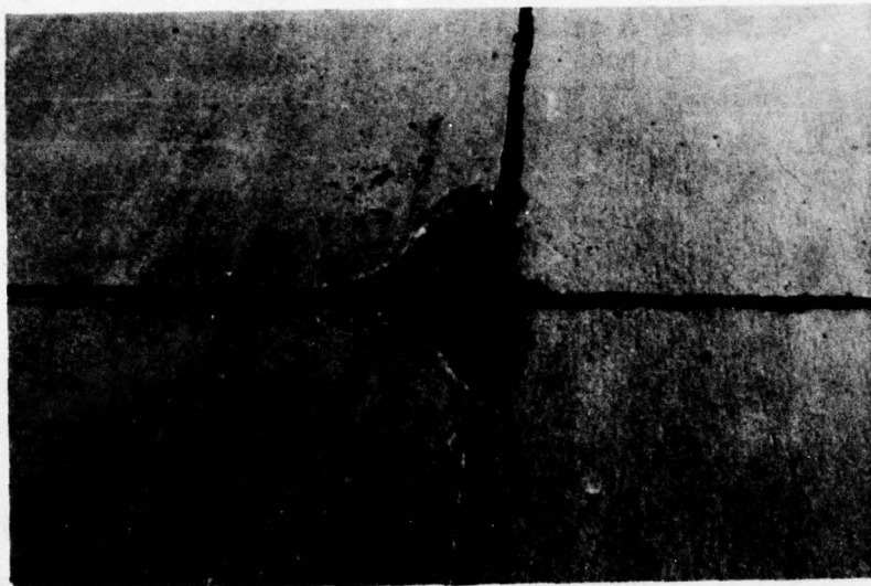
Figure 97. Low Severity Small Patch.
