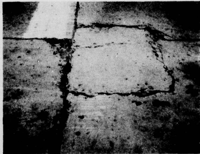
Figure 105. High Severity Patch.
