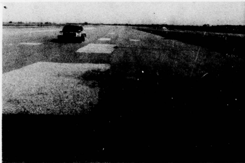
Figure 48. Light Severity Patch With Medium Severity Portion.
