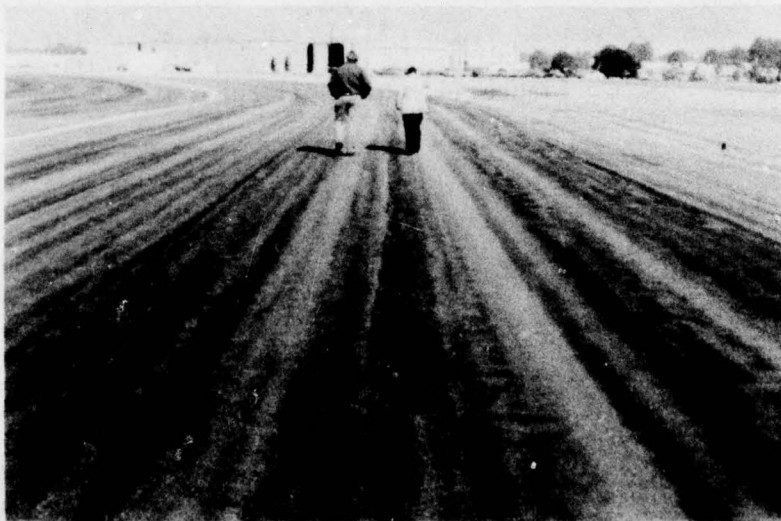
Figure 46. Light Severity Patch.
