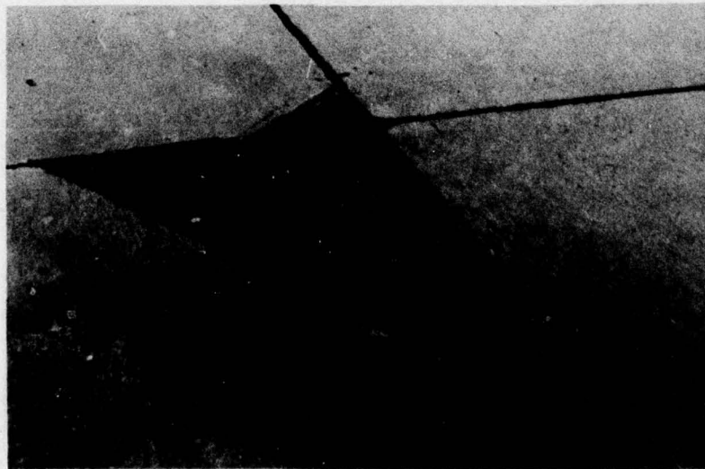
Figure 101. Low Severity Patch.
