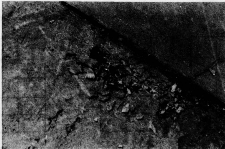
Figure 114. Close-Up of High Severity Scaling.
