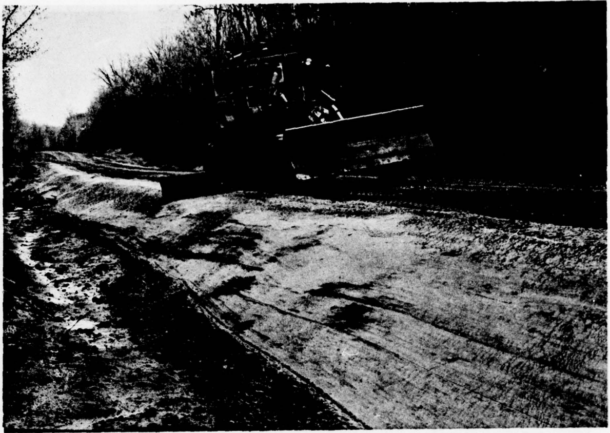
11. Ontonagon County. North Firesteel Road. Second grader in slope finishing team shapes shoulder of sand fill without disturbing gravel. The blade of this grader is specifically adapted to this purpose.
