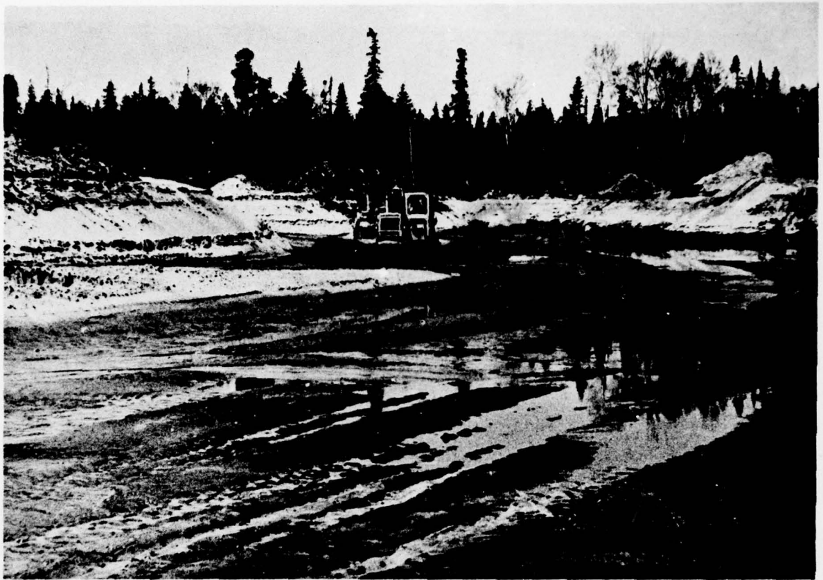
21. Alger County. State Road 28. Although this photo was taken in June 1976, it illustrates the problem of a high ground-water table in the borrow pit which was one of the factors limiting the continuation of earthwork construction through the winter on this project.
