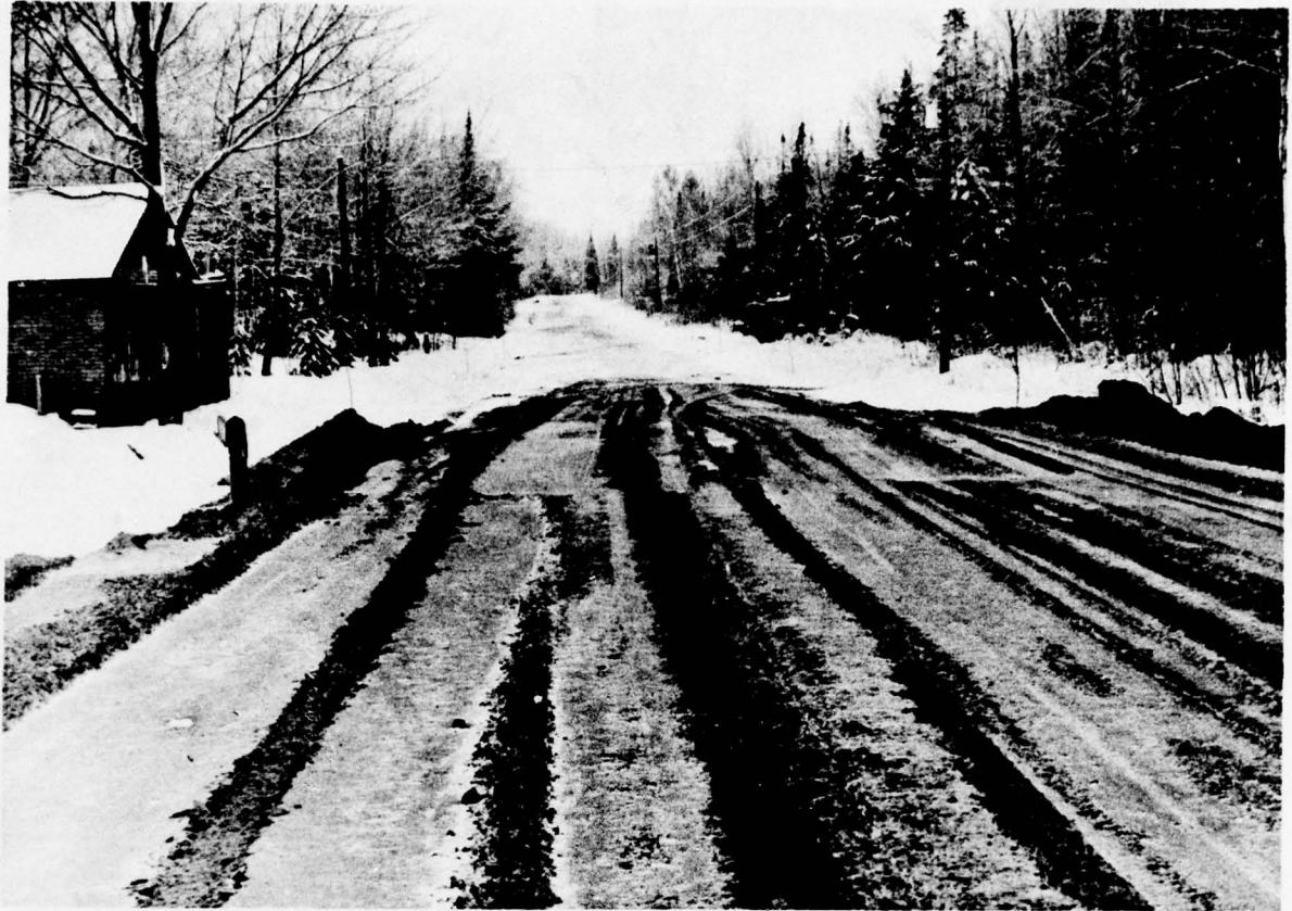
19. Ontonagon County. Cherry Lane. Typical ramp constructed at end of each day's operation. Compacted sand freezes quickly enough that cars and small trucks have little difficulty travelling on fresh grade.
