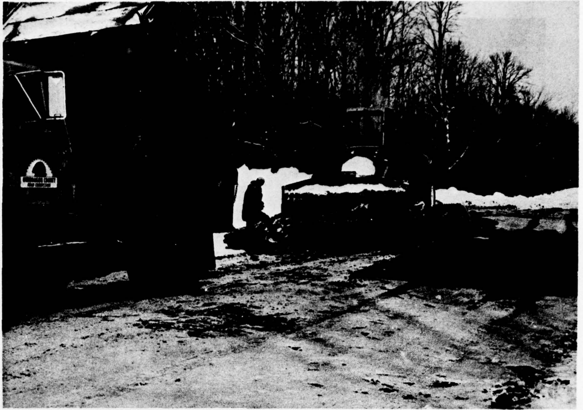
5. Ontonagon County. North Firesteel Road. Spreading of fill with rubber-tired dozer. Note ramp to accommodate occasional local traffic.
