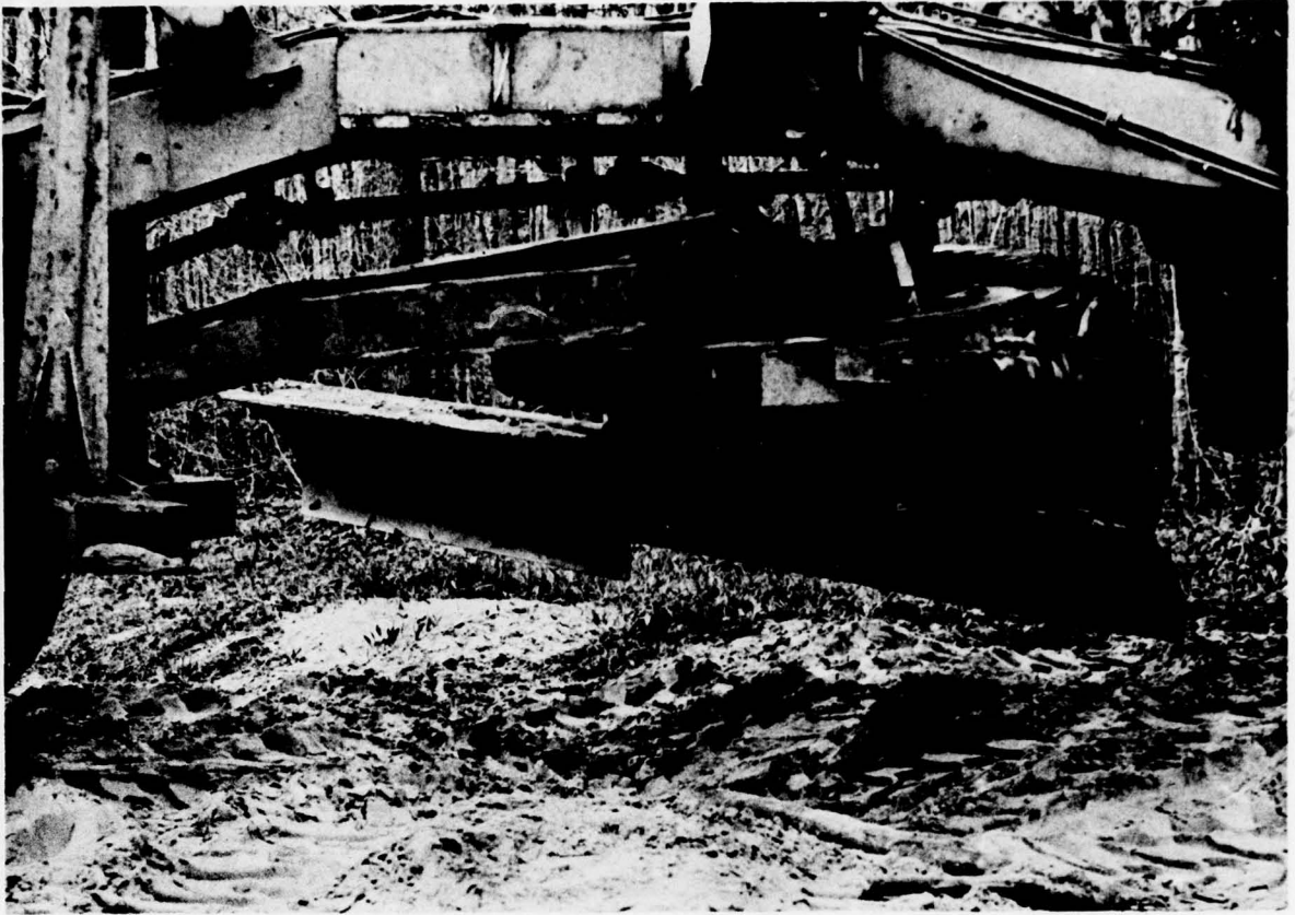
13. Ontonagon County. Detail of blade on second grader of slope finishing team. This arrangement permits shaping the shoulder of the fill without disturbing the gravel traffic course.
