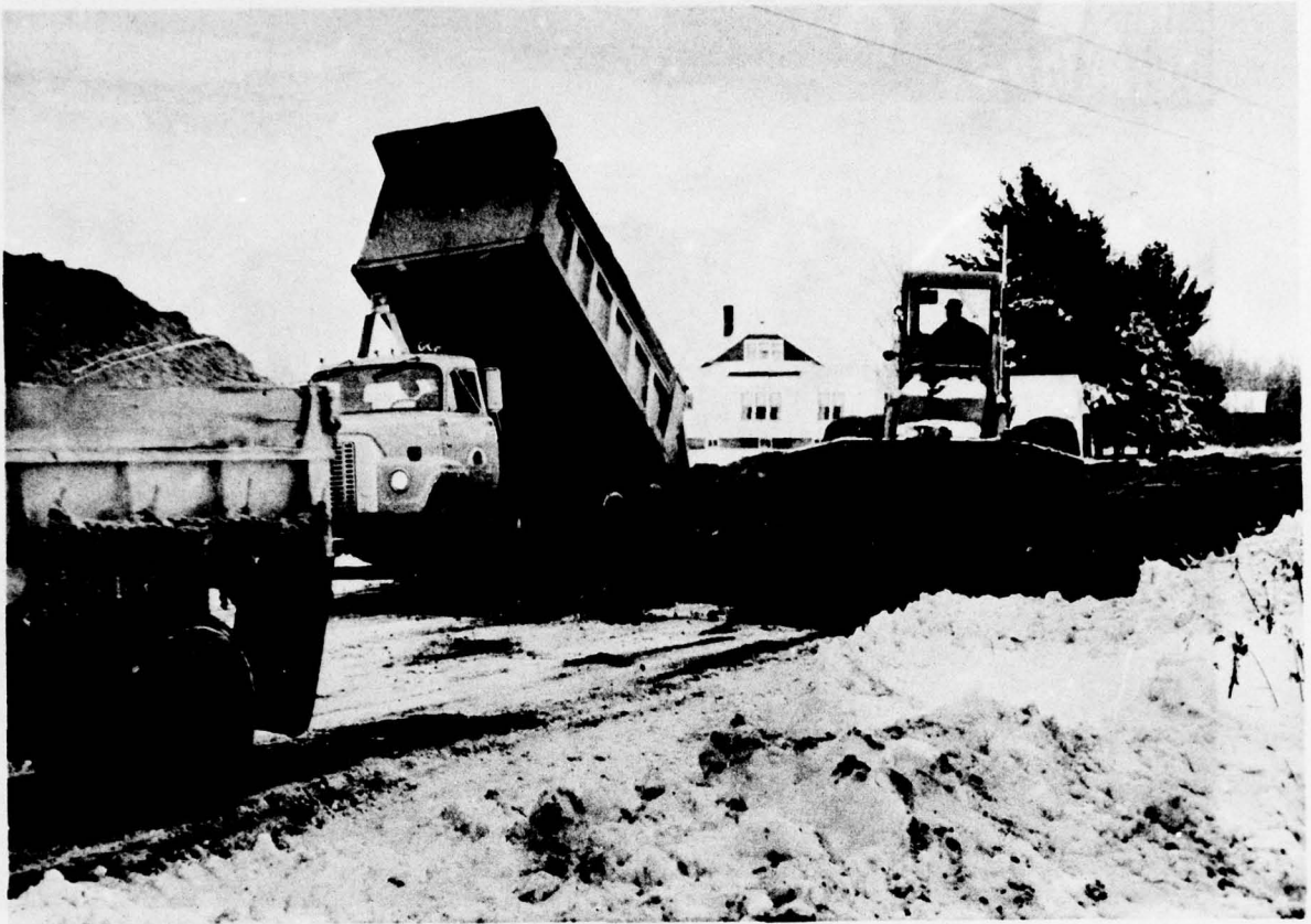
17. Ontonagon County. Wagner Road. General view of hauling, dumping, spreading and compacting.
