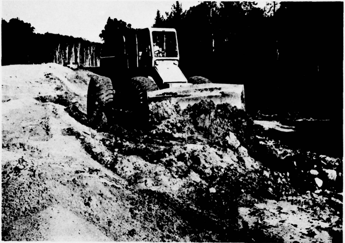
28. Alger County. State Road 28. Large rubber-tired dozer compacting soil in slope zone outside of structural core of sand. See also Photos 25, 26 and 27. Photo taken in June 1976.
