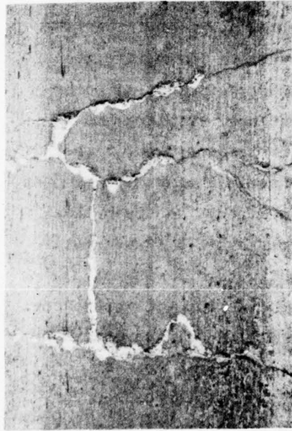
a. Connecting cracks have formed and spalling has begun
