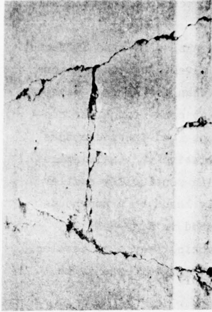
b. Spalling is progressing and pumping has begun
