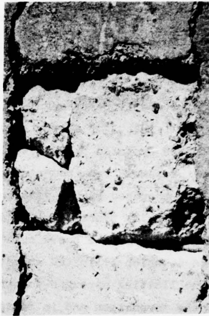
c. Pavement is now broken into several chunks
