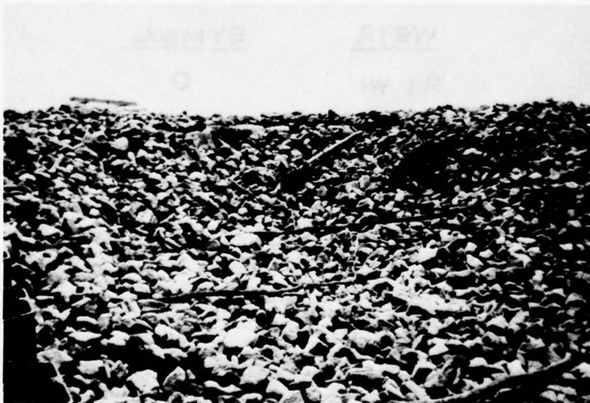
Figure 16. Bank distress at Reach 1 - Weir 2
