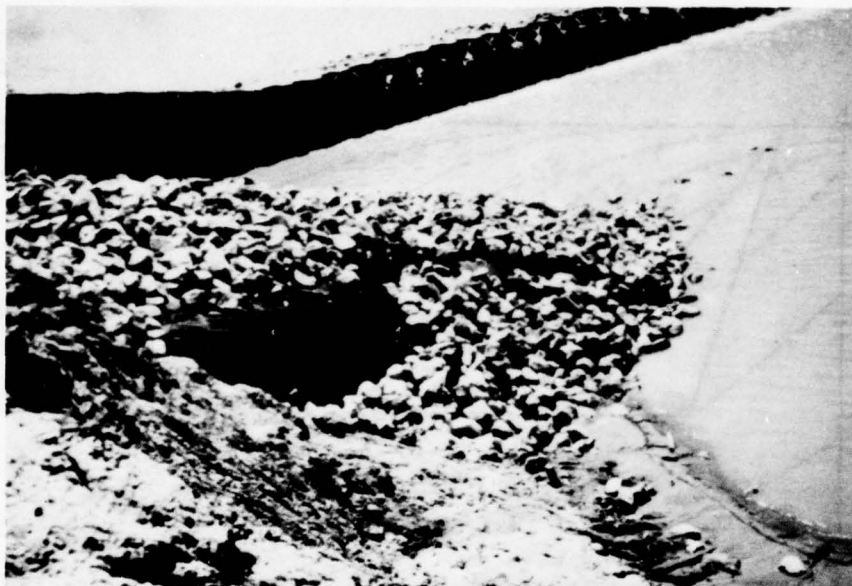
Figure 15. Erosion at downstream edge of riprap Reach 2 - Weir 3
