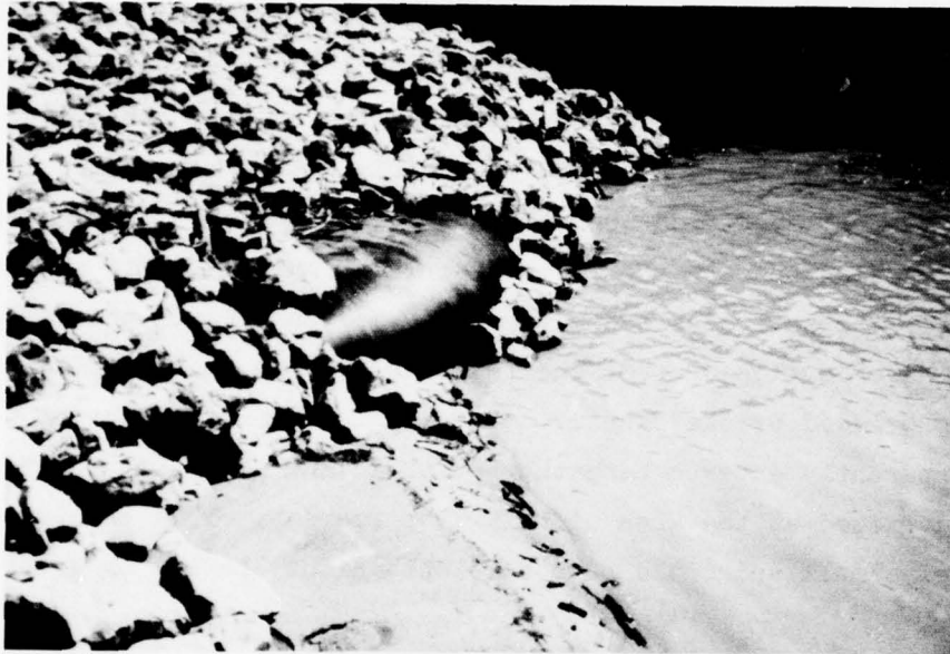
Figure 17. Bulging of filter fabric Reach 2 - Weir 3
