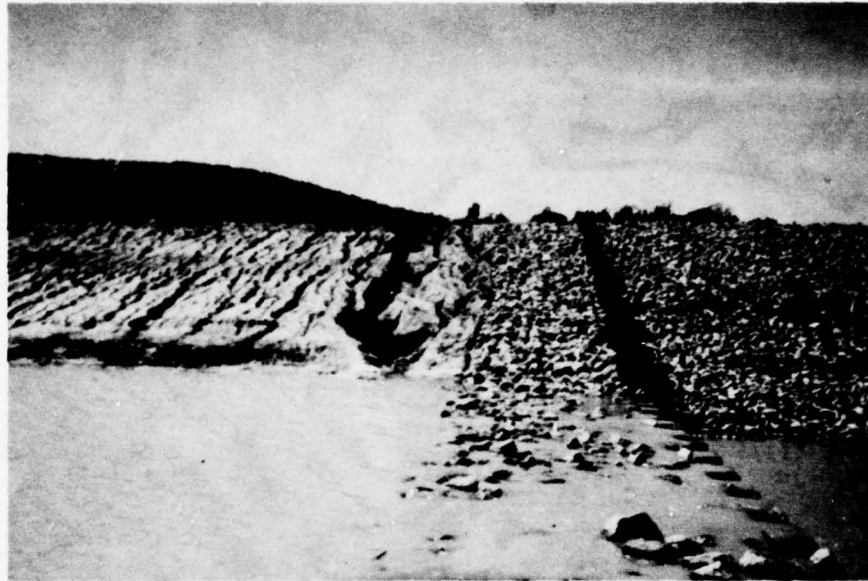
Figure 10. Erosion in unprotected bank Reach 2 - Weir 3
