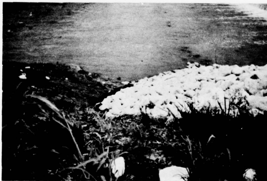
Figure 13. View of "vee" at downstream edge of riprap. End sill is visible just at water surface across channel
