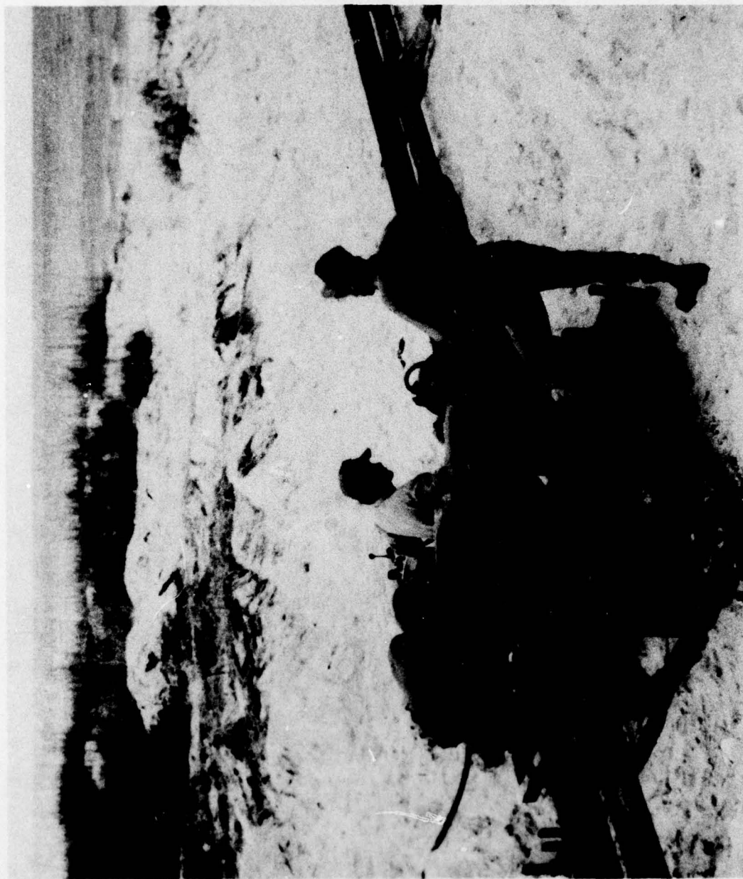
Figure 3. Powered tongs for assembly of present tactical pipeline facility.
