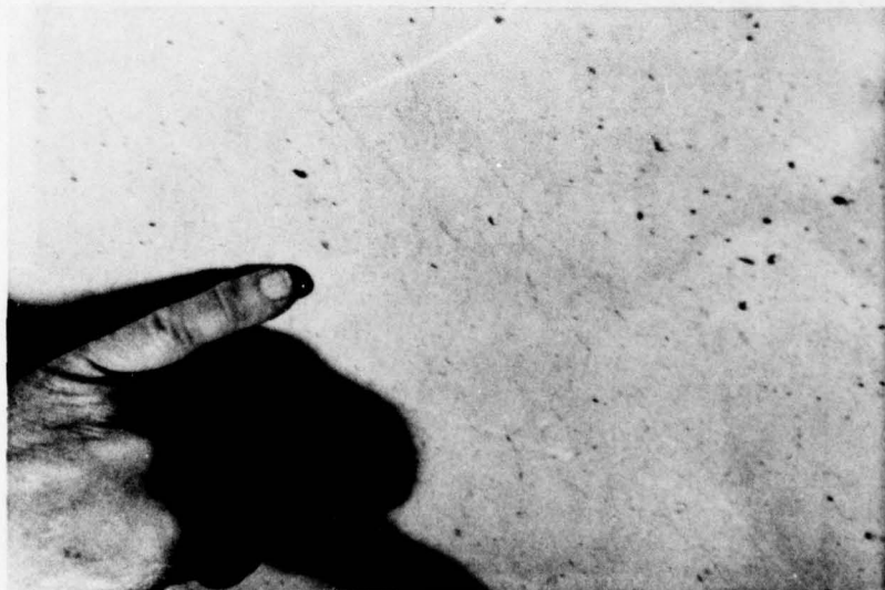
Figure 11. Refractory wear in furnace section 2.
