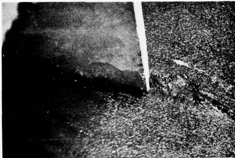
7. 13 Dec 77. Spalled concrete at pedestal/ogee crest construction joint.
