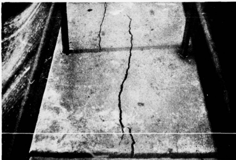
6. 13 Dec 77. Longitudinal cracking of overflow structure walkway - fifth bay from left bank.
