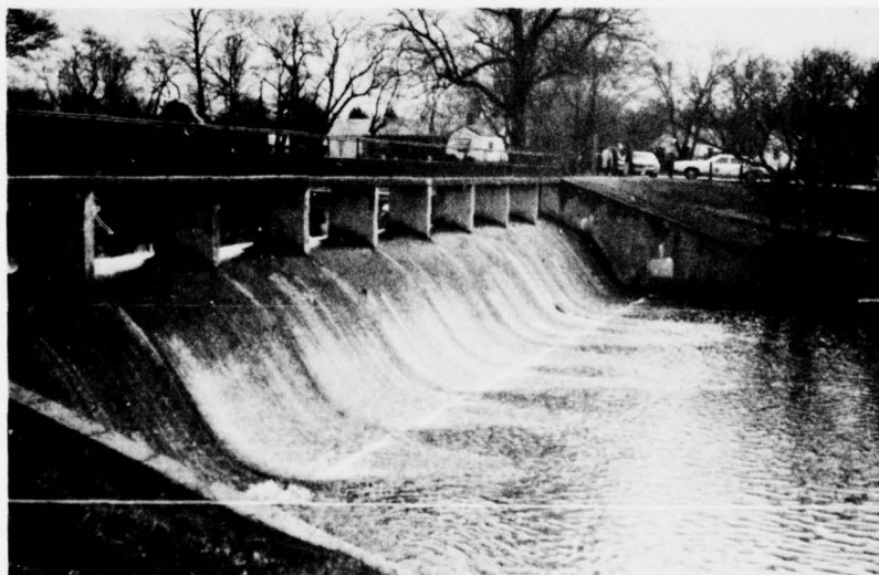
4. 13 Dec 77. Overview of concrete gravity overflow structure, looking east from right abutment wall toward left abutment wall.
