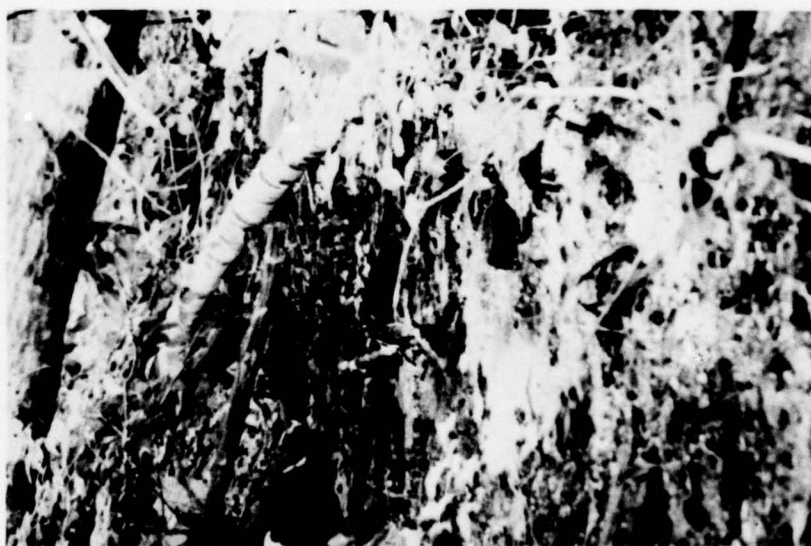
Photo 5 - View of seepage right side of dam.
