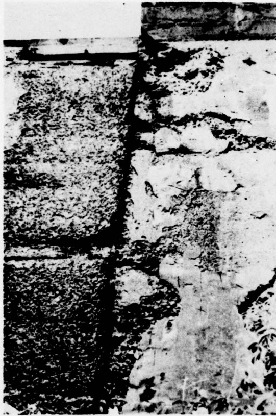
Photo 7 - Construction joint and spalling left side of notch spillway.
