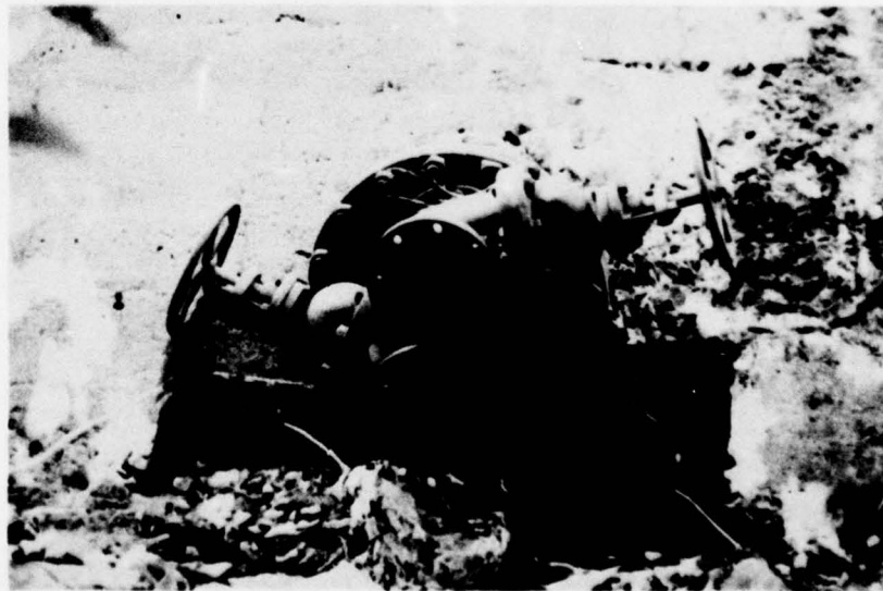
Photo 8 - View of two 6-inch valves installed on flange plate on plugged 18-inch cast iron pipe.
