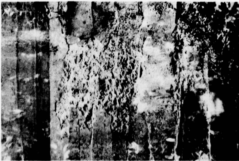
Photo 7 - Typical spalling on downstream face of dam.
