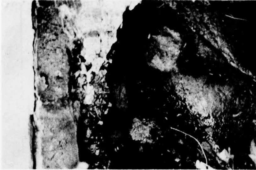
Photo 8 - Concrete deterioration and leakage over rock outcrop at left abutment.
