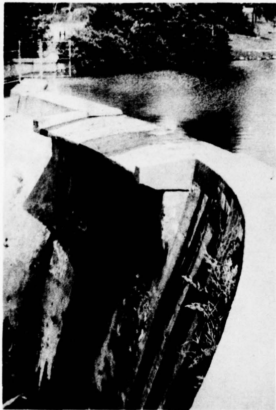
Photo 1 - View along crest of dam from left abutment showing main spillway and service spillway on right abutment.
