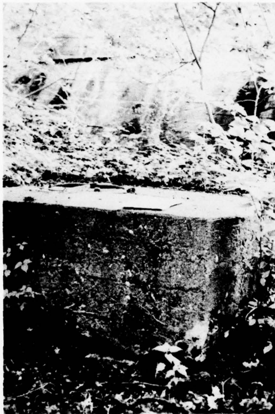
Photo 9 - Concrete valve vault for low level outlet pipe.
