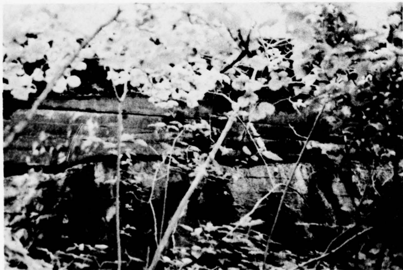
Photo 8 - Horizontal crack right side near abutment.
