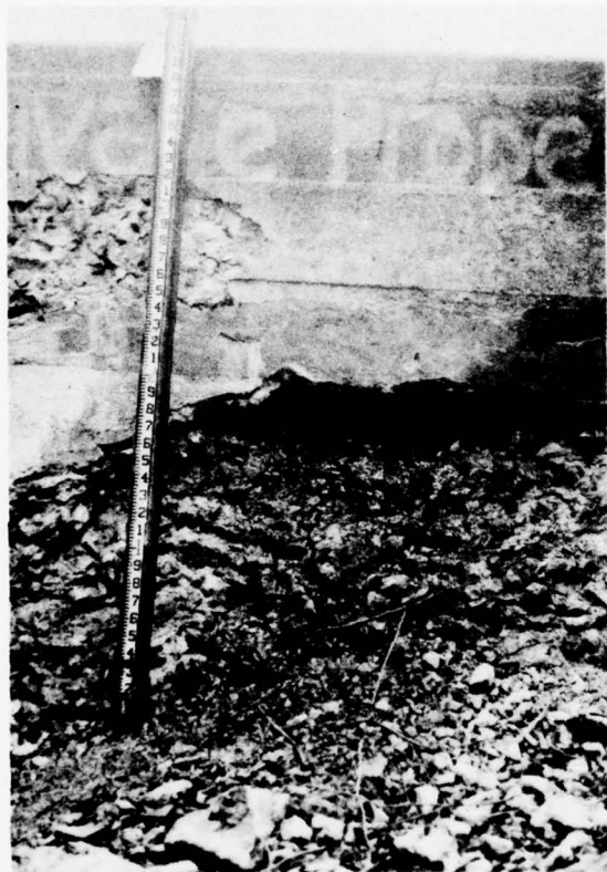
Photo 7 - Spalling and leakage near left abutment.
