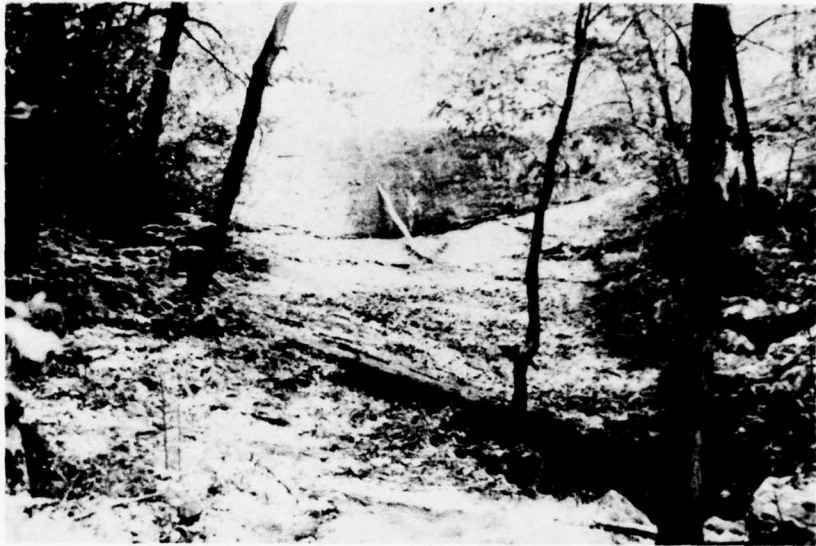
Photo 3 - View of dam and spillway from downstream showing concrete apron and plunge pool below spillway.
