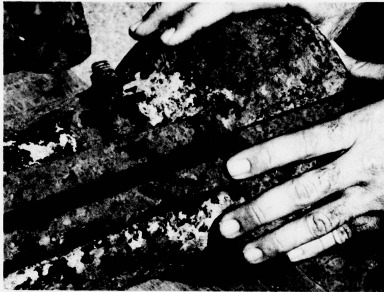
Figure 9. Corroded Hi-Shear steel fasteners slipping through the pipe flange.
