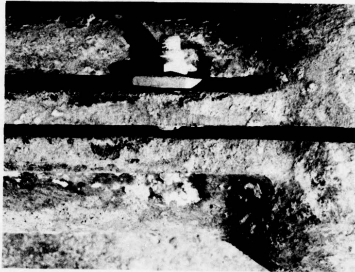
Figure 7. Gap in pipe halves due to slippage of Hi-Shear stainless steel fasteners.
