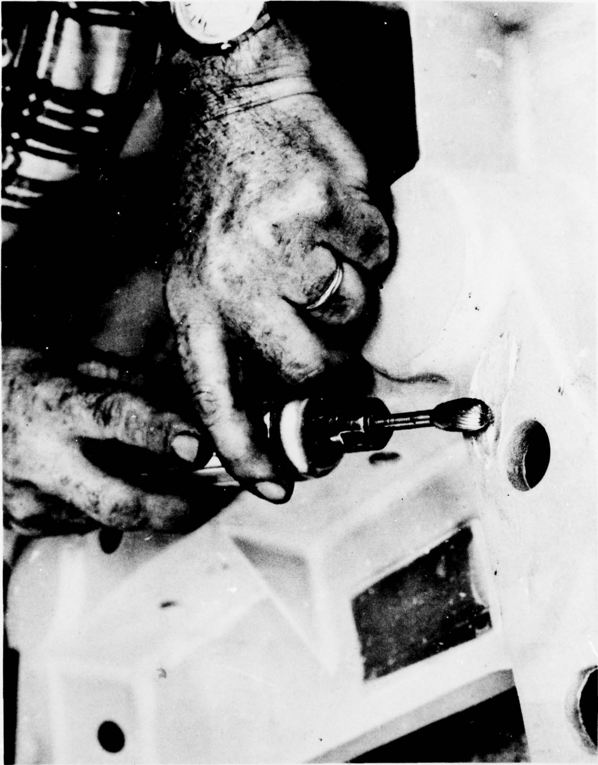
FIGURE 145 USE OF A FINE TOOTH ROTARY FILE FOR WELD BEAD REINFORCEMENT REMOVAL
