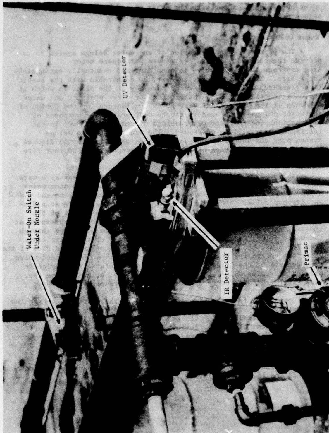
FIGURE 4. DETECTORS MOUNTED IN END OF CONVEYOR
