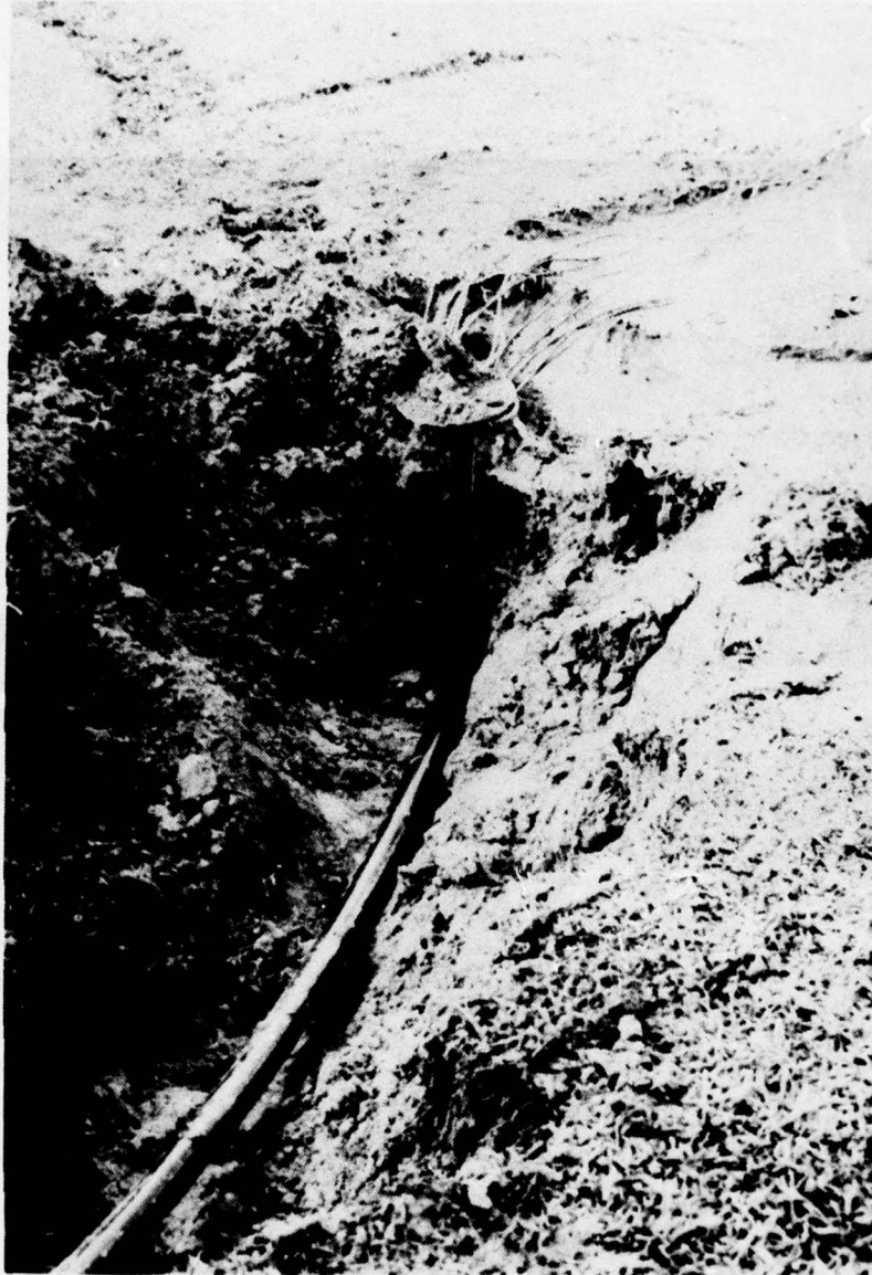
Figure 11. Anode Lead Wires Running From Well Cap
