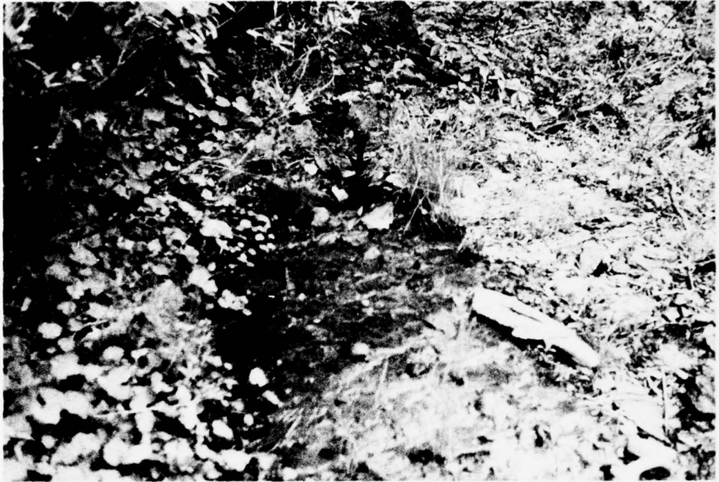
PHOTO 5 Clear Seepage 36' Downstream of Spillway
