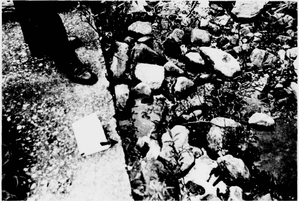
PHOTO 4 Clear Seepage at End of Spillway Bucket
