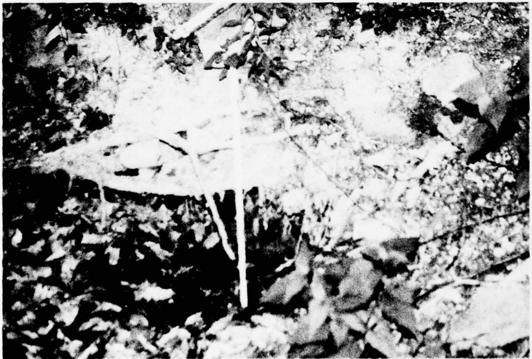
PHOTO 6 Clear Seepage at Toe of Spillway Below Intake Tower (appx. 100 g.p.m.)
