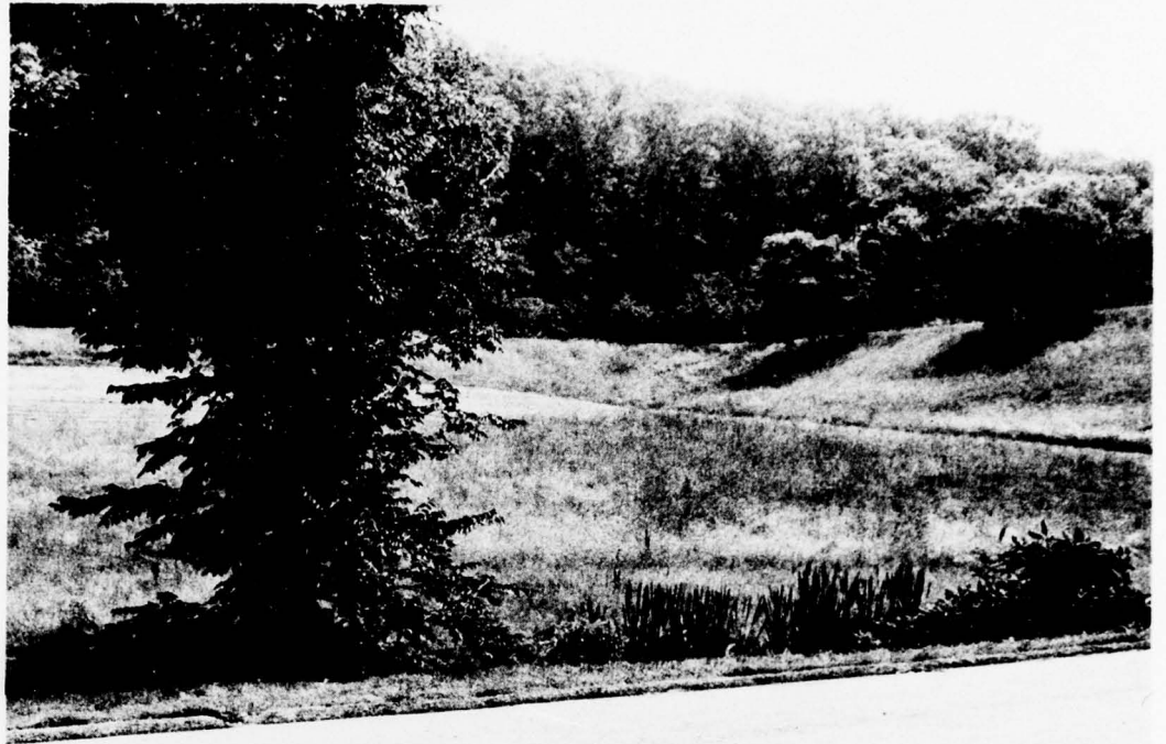
PHOTO 7. Swampy Area Just Downstream From Toe on Right Side of Embankment (150 Feet by 100 Feet)
