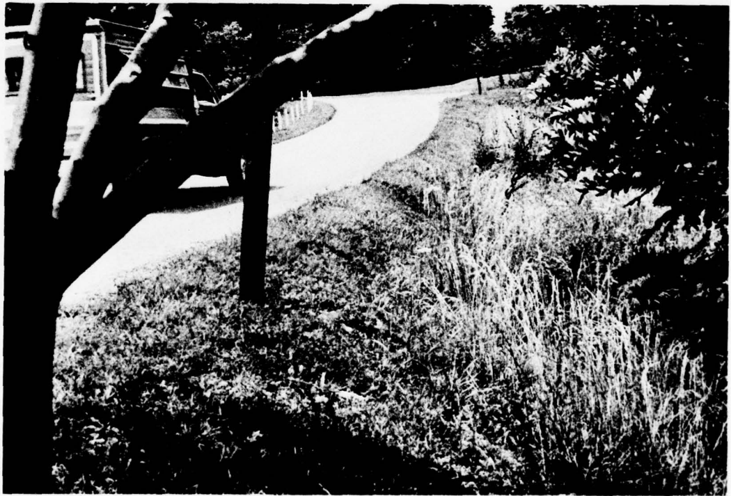
PHOTO 6. Location of SLoughing at Top of Downstream Face (Looking Left)
