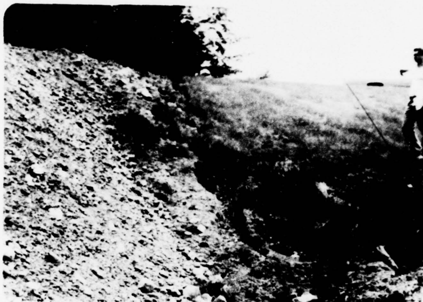
EROSION ON DOWNSTREAM EMBANKMENT SLOPE
