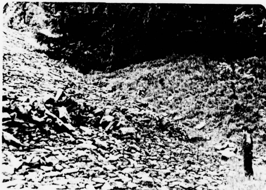
Photograph No. 6 Typical bulges in downstream face riprap.
