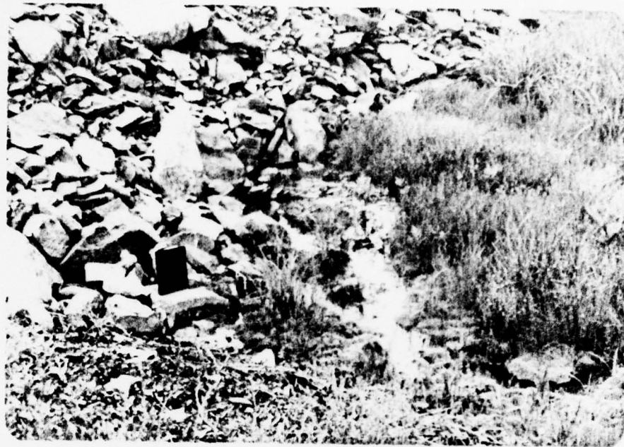
Photograph No. 7 Seepage at toe.
