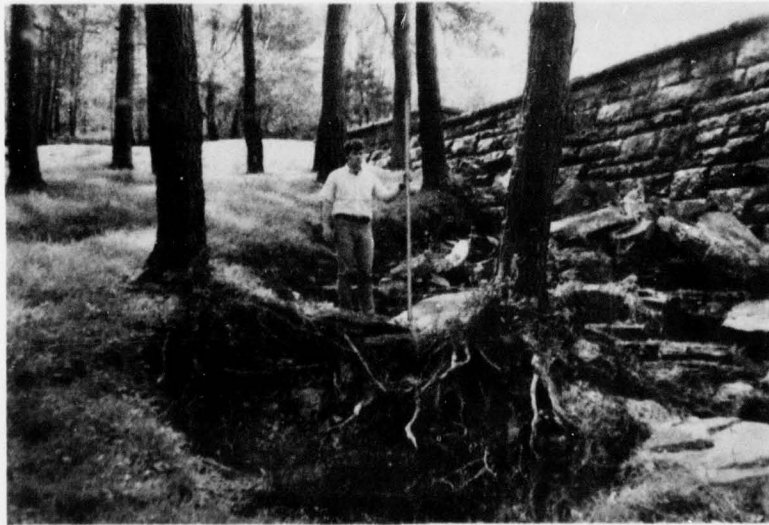
H. Eroded Area Downstream from Right Auxiliary Spillway
