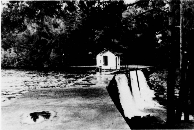
A. Top of Dam and Auxiliary and Main Spillways. Access to Gatehouse is Plank Footbridge Over Main Spillway.
