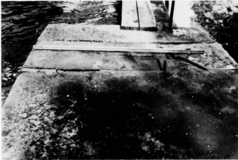
E. Broken Capstone and Missing Mortar at End of Right Auxiliary Spillway
