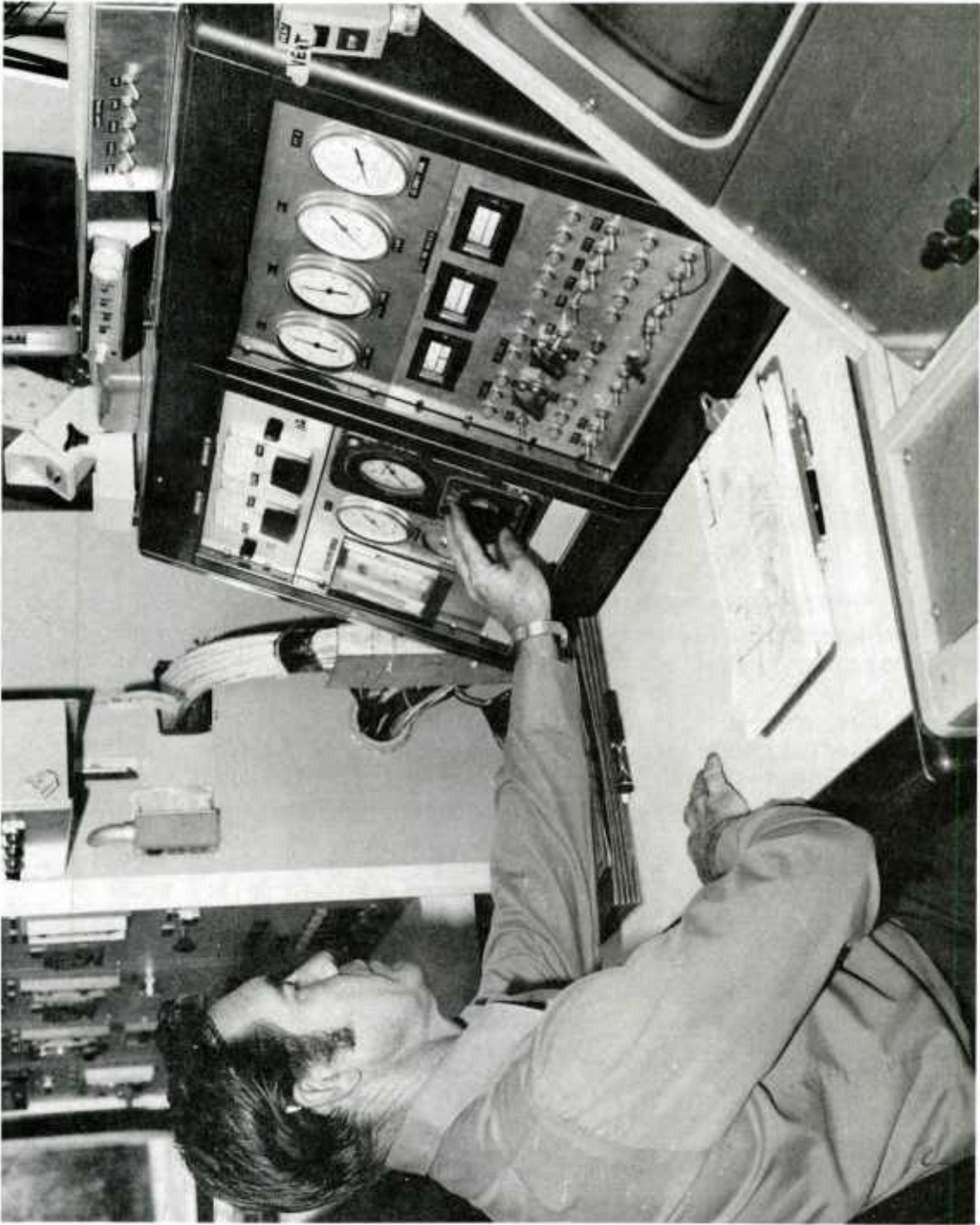
Figure 7. Control panel for slurry preparation and feed system.
