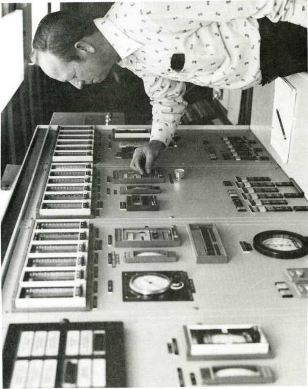
Figure 8. Incinerator instrumentation and control panel.
