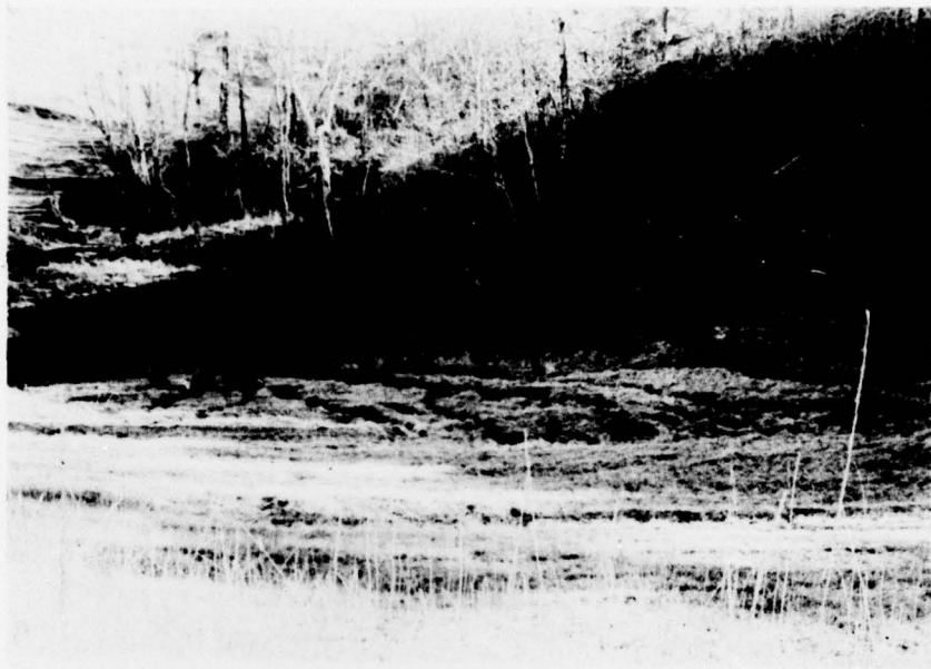
VIEW LOOKING DOWNSTREAM FROM CREST OF DAM - NOTE EROSION ON THE DOWNSTREAM SLOPE
