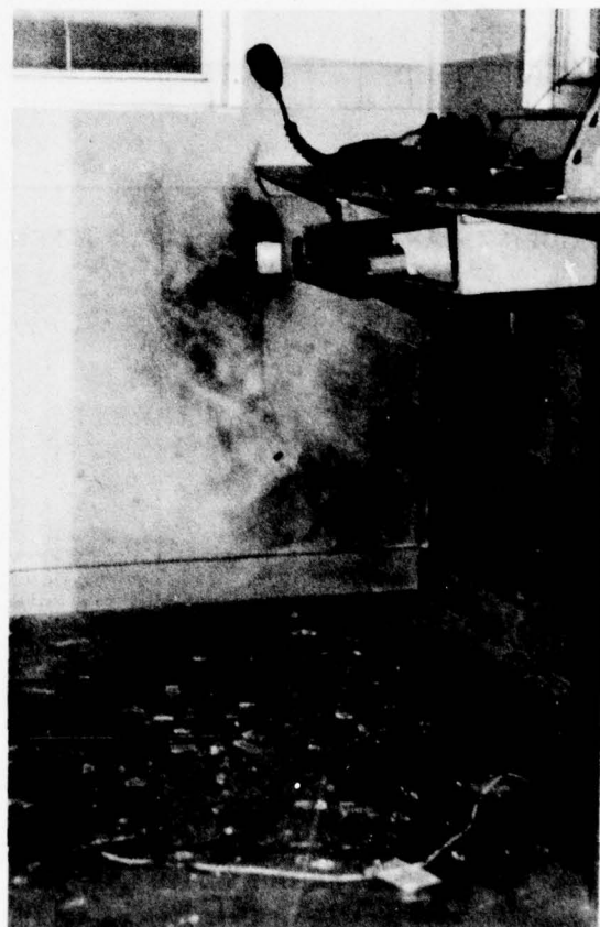
FIGURE 7. EXPLOSIVE DAMAGE IN GUARD SHACK.
