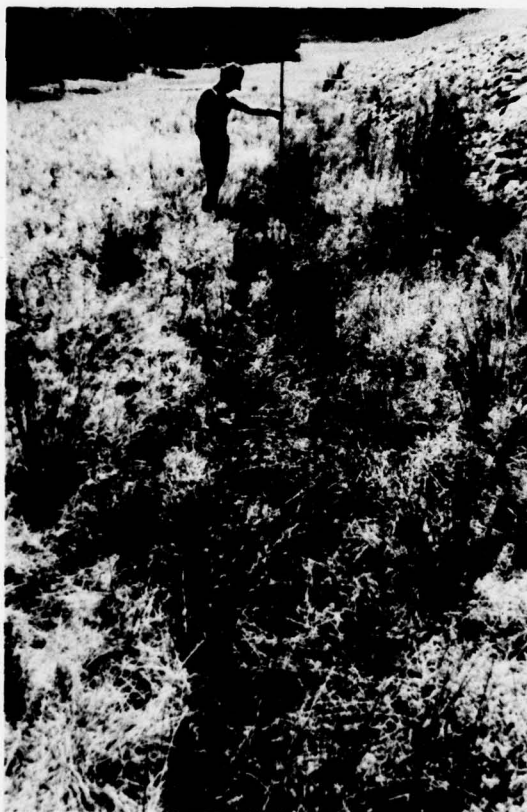
F. Wet Area at the Downstream Toe of Embankment.
