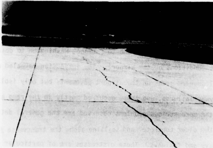
Figure A-43 - Reflective Crack Through Concrete Slab on an Econocrete Subbase, Shreveport.
