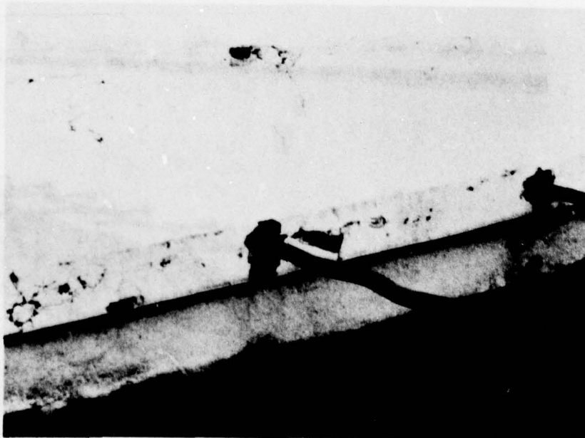
Figure A-23. View of Keyway with Second-Half of Wiggle Bolt in Place, Detroit.
