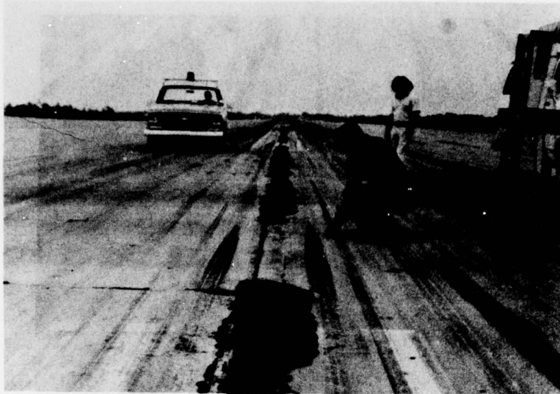
Figure A-36 - Longitudinal Keyed Joint Distress and Repair, Indianapolis.
