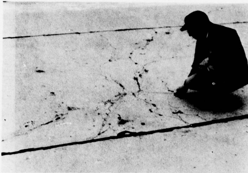
Figure A-38 - Concrete Deterioration, Indianapolis.
