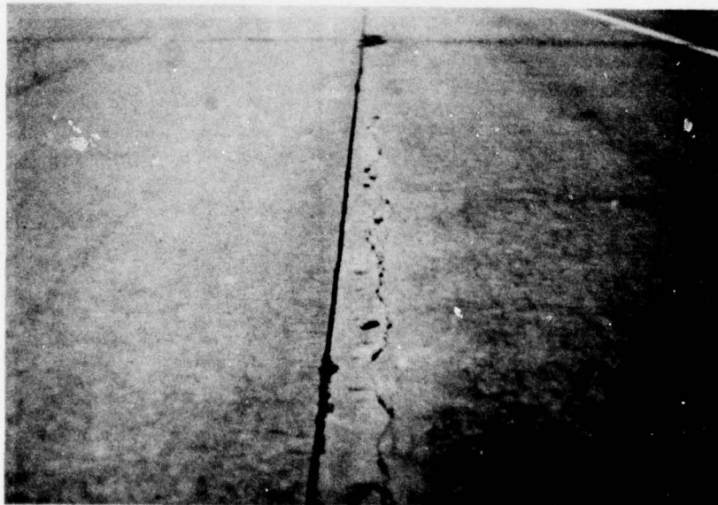
Figure A-14. Longitudinal Joint Distress Between Transverse Joints, Stapleton Airport.
