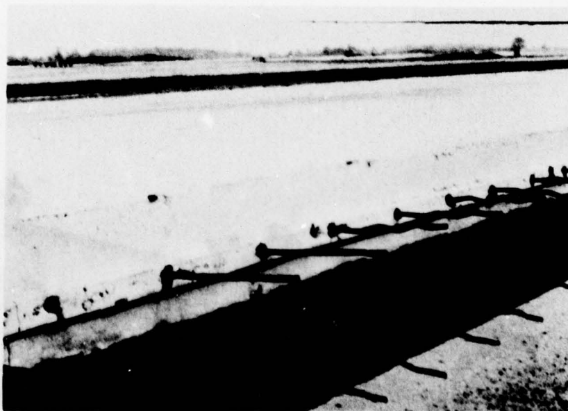
Figure A-24. Further View of Keyway and Wiggle Bolts in Place, Detroit.
