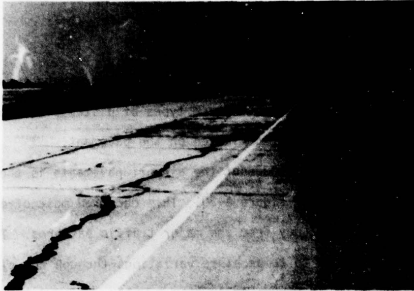
Figure A-30 - Longitudinal Cracking, Kansas City.
