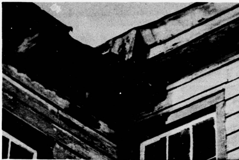
A) Deteriorated Roof Junction, Section D-1 and B (West Elevation of B)
