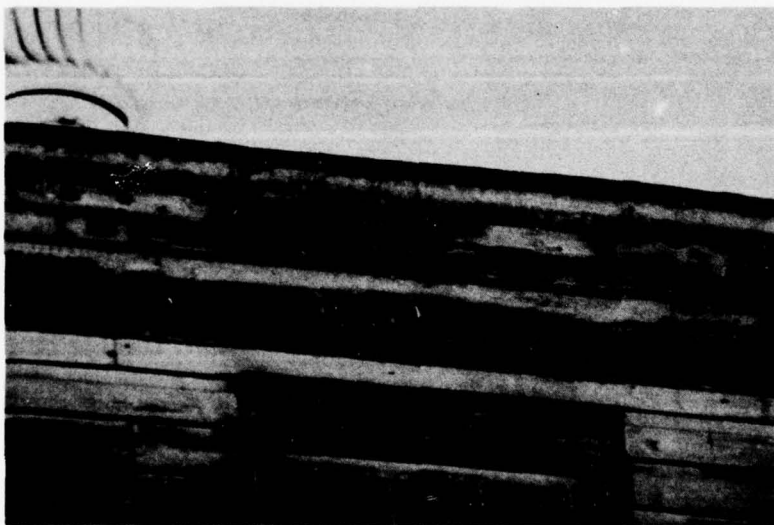
B) Deteriorated Cornice, Section B, West Elevation
