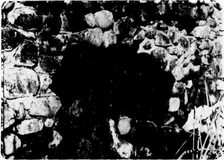
Bulge collapse and loss of interior portion of downstream face of dam.
