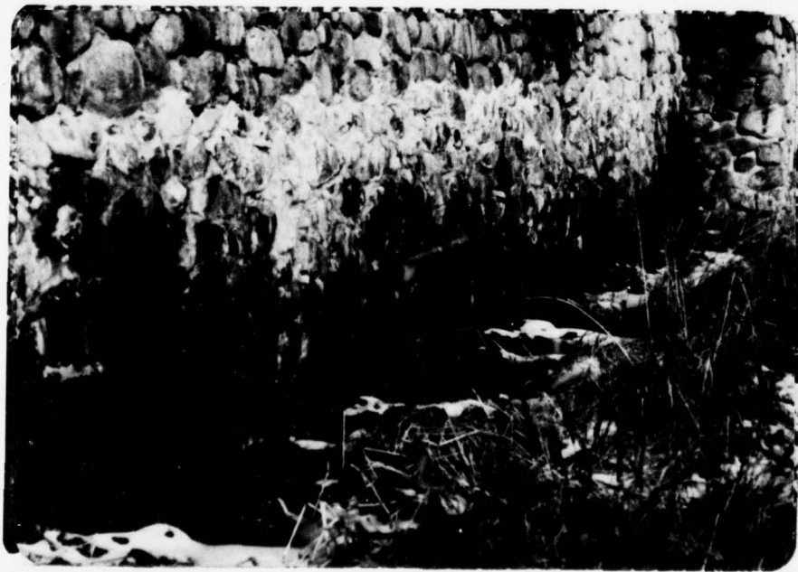
Seepage along downstream face of cobble-faced masonry dam.
