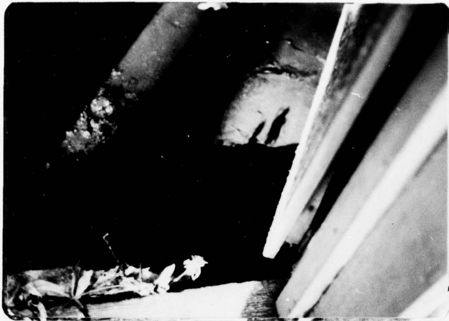
Clear water flowing from hole in concrete floor of former pump house.
