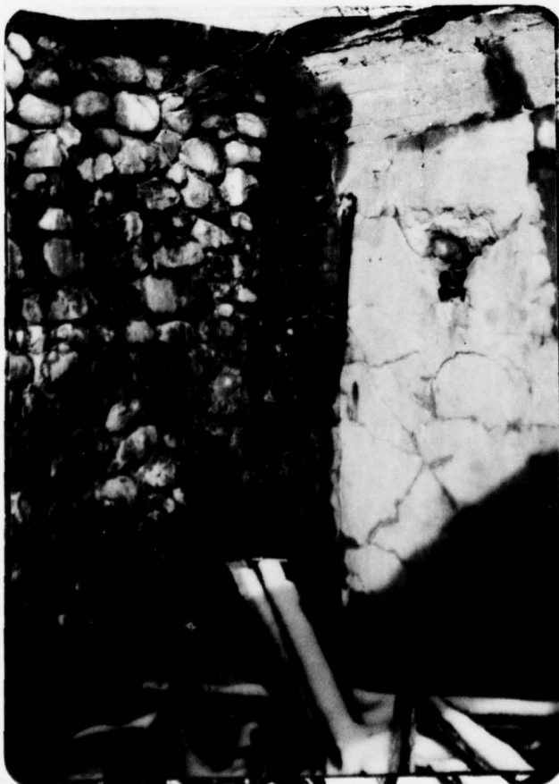
Seepage at downstream face of dam in abandoned generator house.
