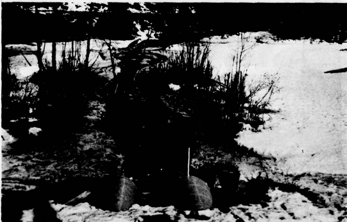
TWO 72 INCH CULVERTS ON CALIFORNIA CREEK CROSSING ALYESKA HIGHWAY. NOT OF SUFFICIENT SIZE TO CARRY INTERMEDIATE REGIONAL FLOOD
