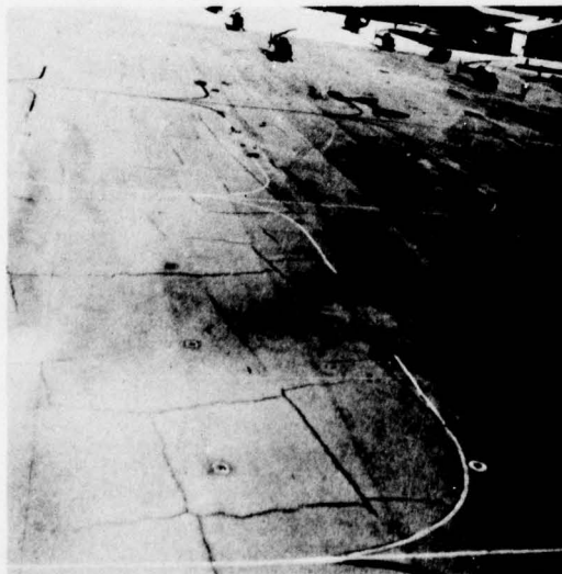
Photo 20. Fort Stewart--crack pattern from soil-cement base
