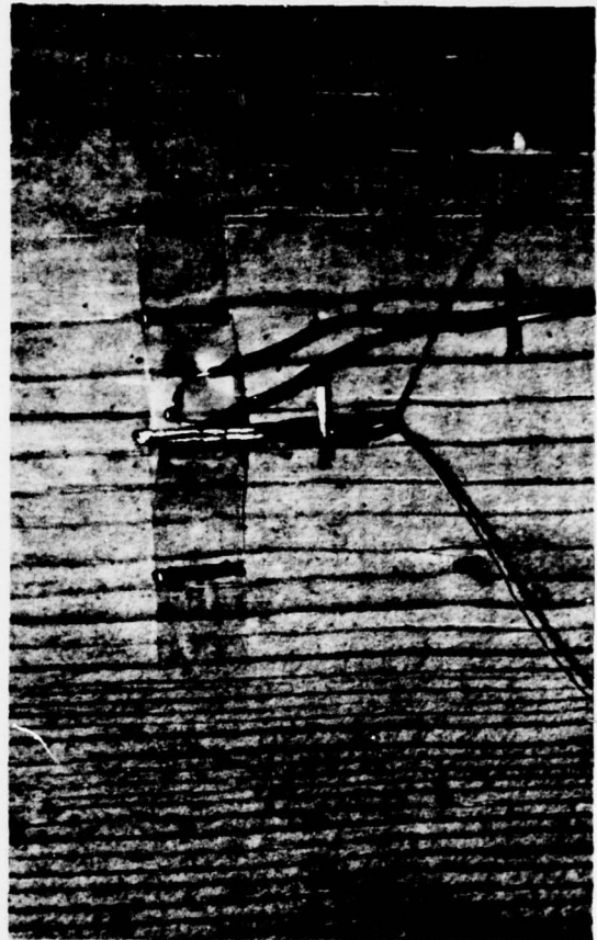
Figure 5. - - Moisture probe and thermocouple attached to interior surface of sheathing board. (M 144 309)
