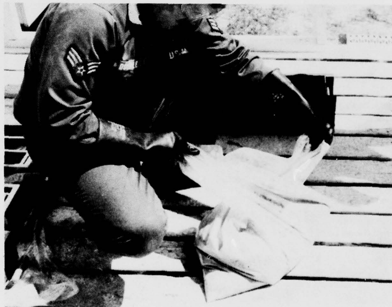
Figure 12 Closing the Mixing Bag Leaving Only a Small Space Above the Polymer Mortar
