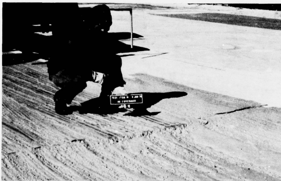
Figure 25 Lip Created at Edge of Patch by Movement of Crushed Stone
