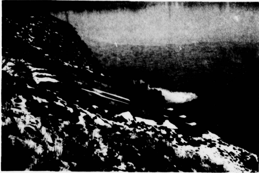
Photo 9 - Outlet pipes from Passaic River pump station. (11-29-78)
