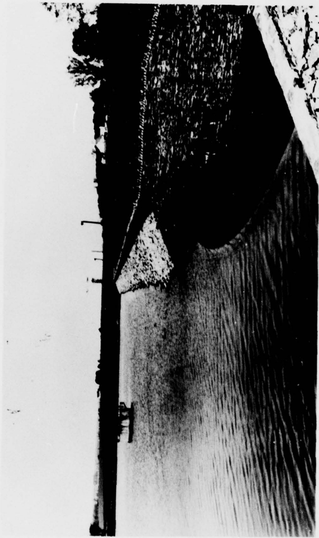
PHOTOGRAPH SHOWS THE FINISHED RIPRAP SLOPE WHICH TERMINATES AT THE BASE OF THE PARAPET WALL. COMPARE THE FINISHED SLOPE SHOWN HERE WITH PHOTOGRAPH NO. 7 WHICH SHOWS THE SETTLEMENT OBSERVED DURING THE INSPECTION.
