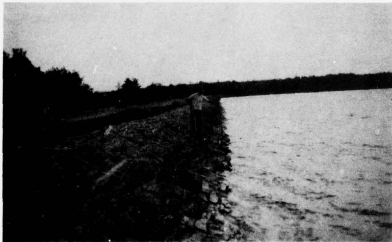
D. Damaged Riprap Near Left Abutment.
