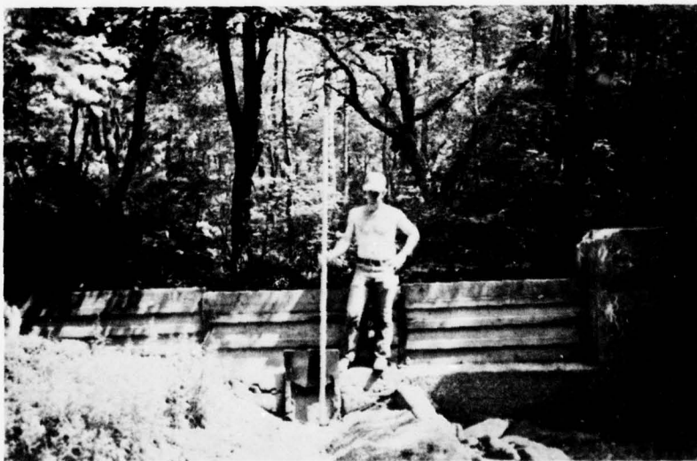
M. Left Side of Diversion Structure — View from Upstream. Original Channel of West West Branch Schuylkill River in Background.
